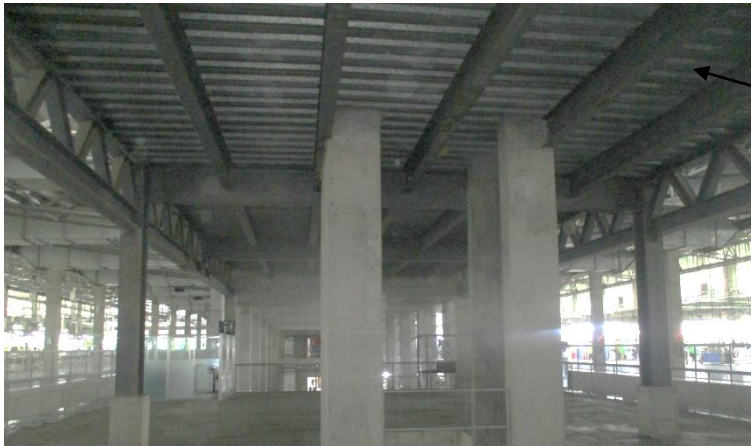
No connection detail was found in drawing for the steel roof structure around the lift.
