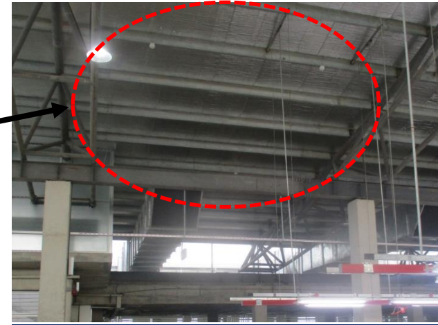
On the marked location, horizontal bracing was not observed
