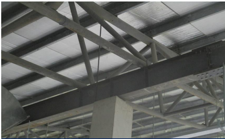
No RC column-steel beam connection detail and sectional detail of steel beam were provided in the as-built drawing.
