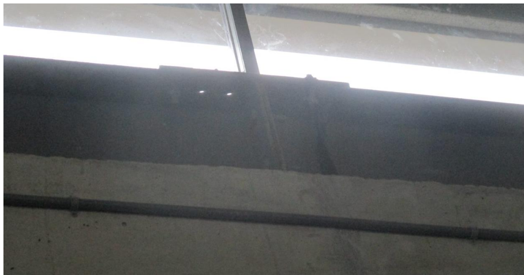
Bolt missing at some splice locations of beam on top floor
