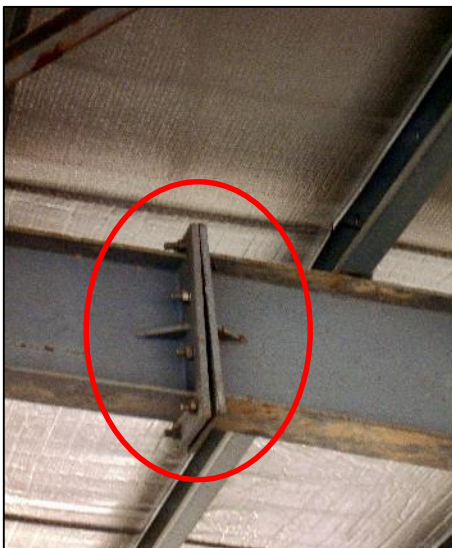
Gap in connection plate
