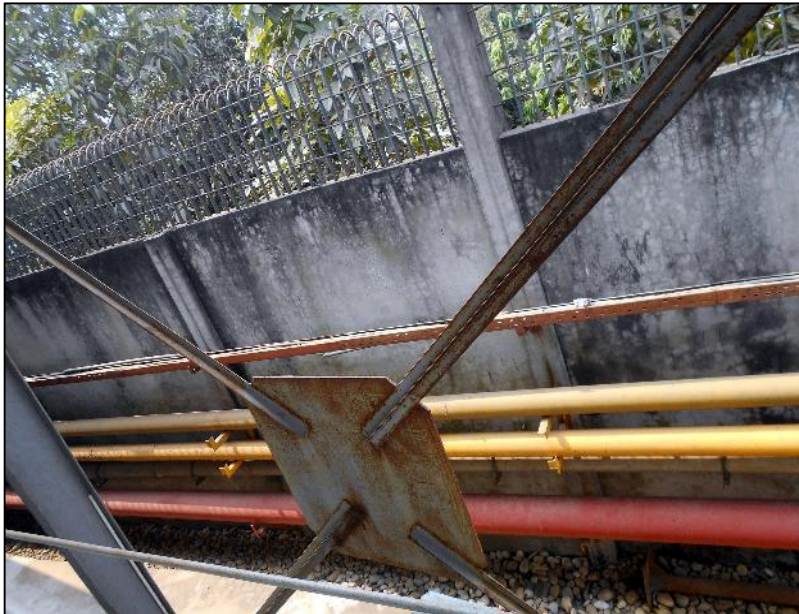
Corrosion in bracing
