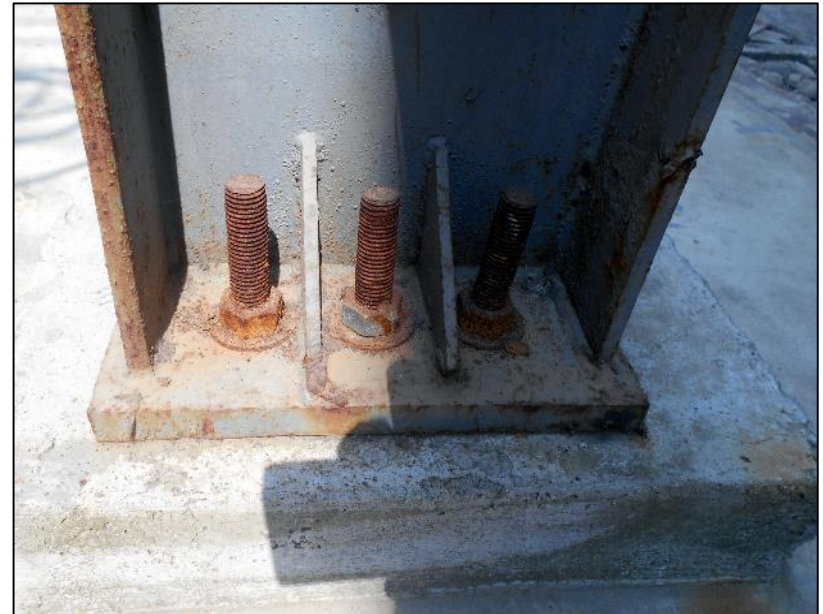
Corrosion in column and bolt
