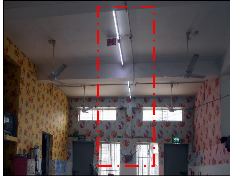
No columns and beam found in the marked location
