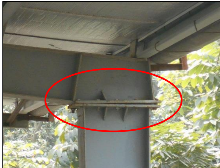
Gap in connection plate
