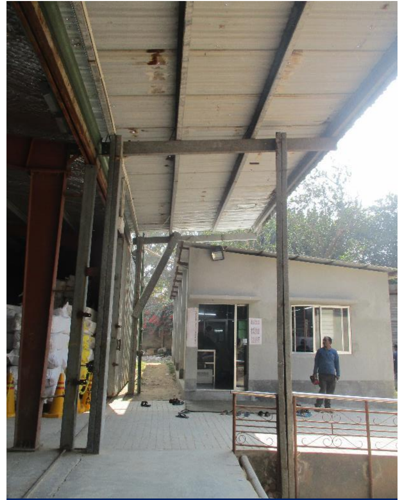
No bracing system
