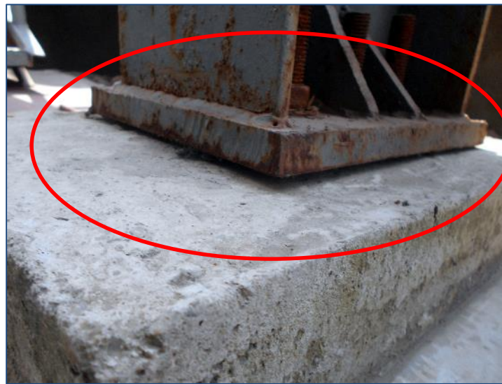
Gap between baseplate and concrete short column
