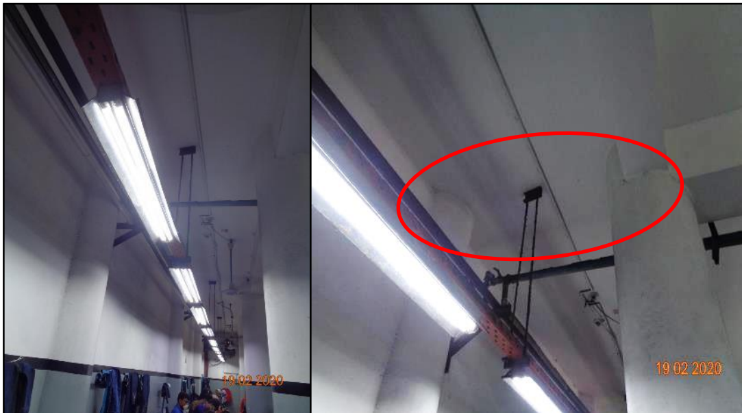
Cantilever beam was not found at 1st floor level
