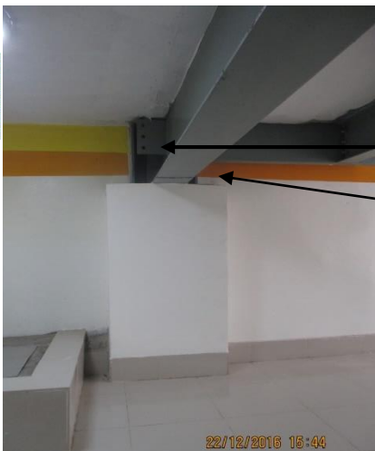
Apparently very poor connection between Column and Beam of Stair-3
