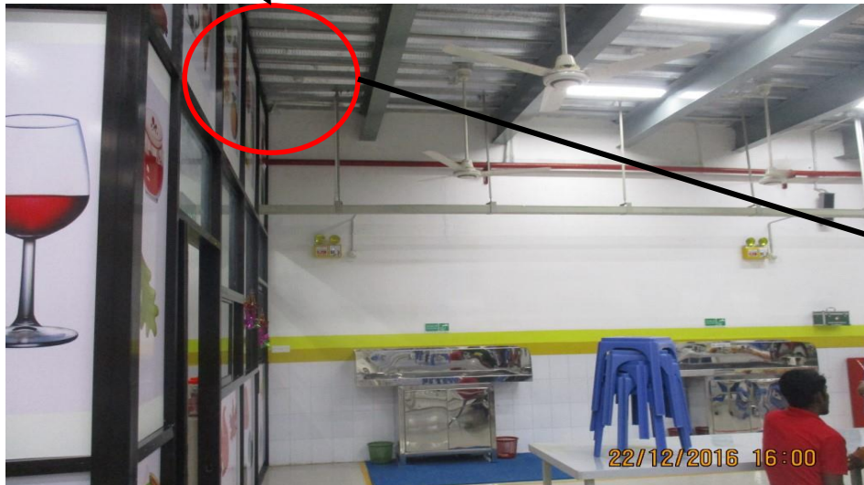
Damage of deck metal sheet was observed near the dining area on ground floor
