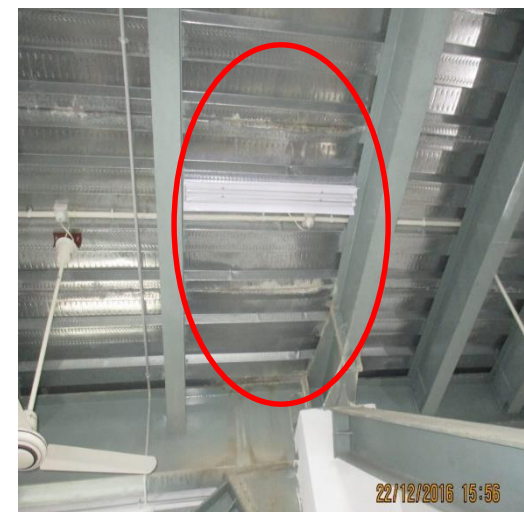
Corrosion was observed on ground floor deck sheet
