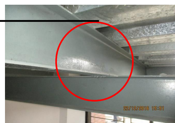
Welded connection was found between main & secondary beam
