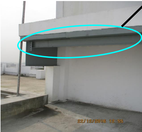
The marked beam was absent in beam layout but that beam was observed under the top slab of stair case-2
