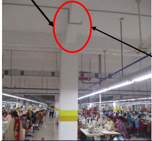
Width of FB-1A beam in red marked area was found 9" instead of 10" in beam schedule
