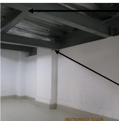
Apparently non engineered connection between two structural members
