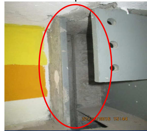
At Column beam connection, no bolt was found
