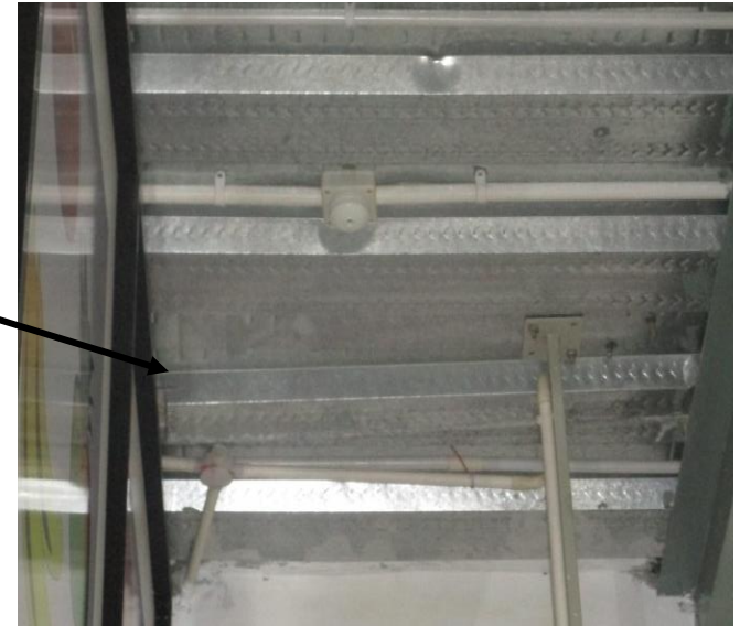
Damaged deck slab
