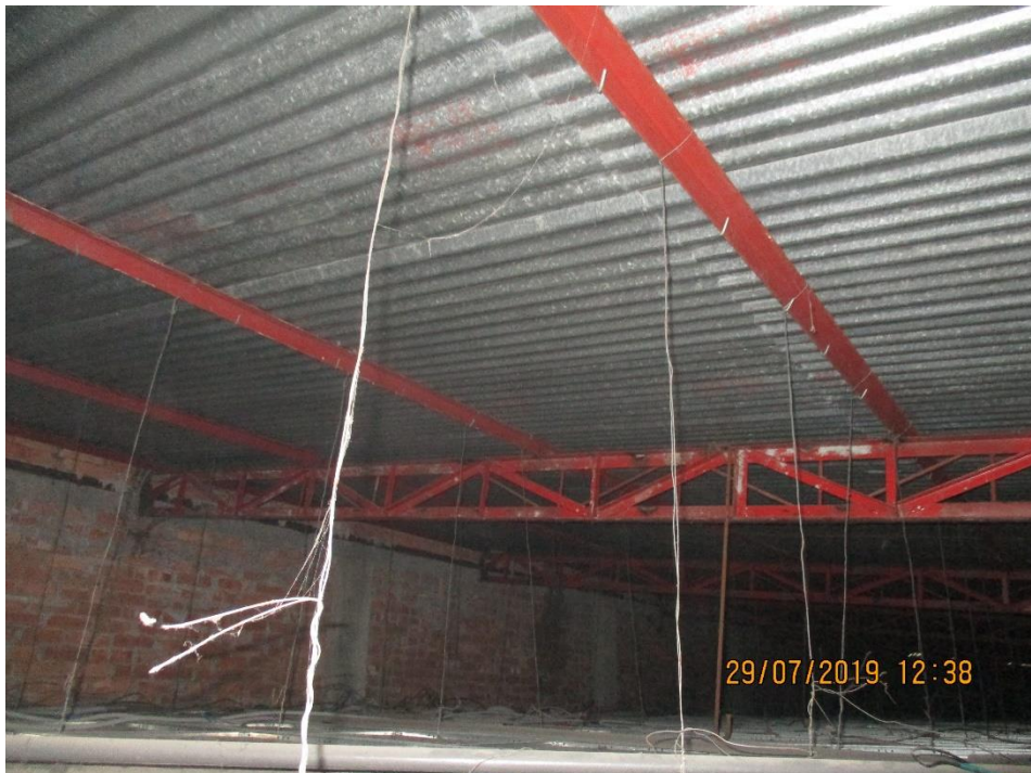
Connection & load path not obvious
