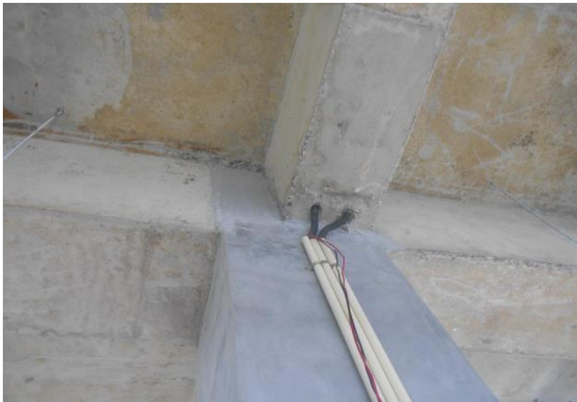
Electrical cable pass through beams.
