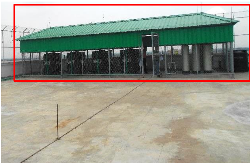
Undocumented steel shed at roof.
