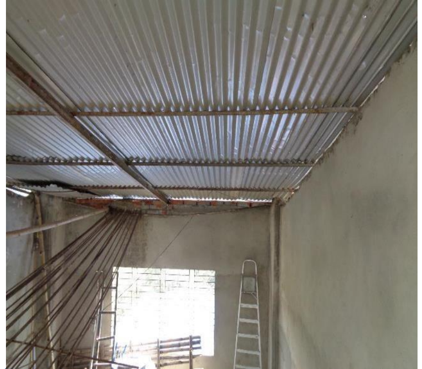
Non engineer steel roof at south stair
