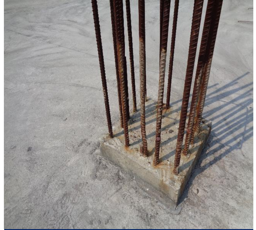
Corrosion in exposed rebar
