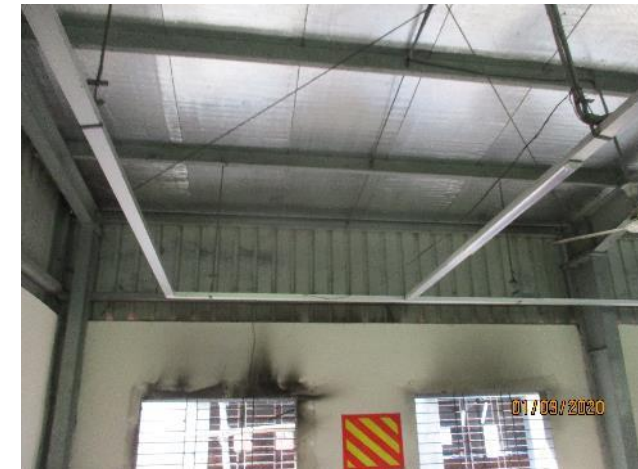
Absence of load transfer member in long direction
