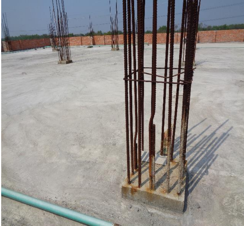
Corrosion in exposed rebar
