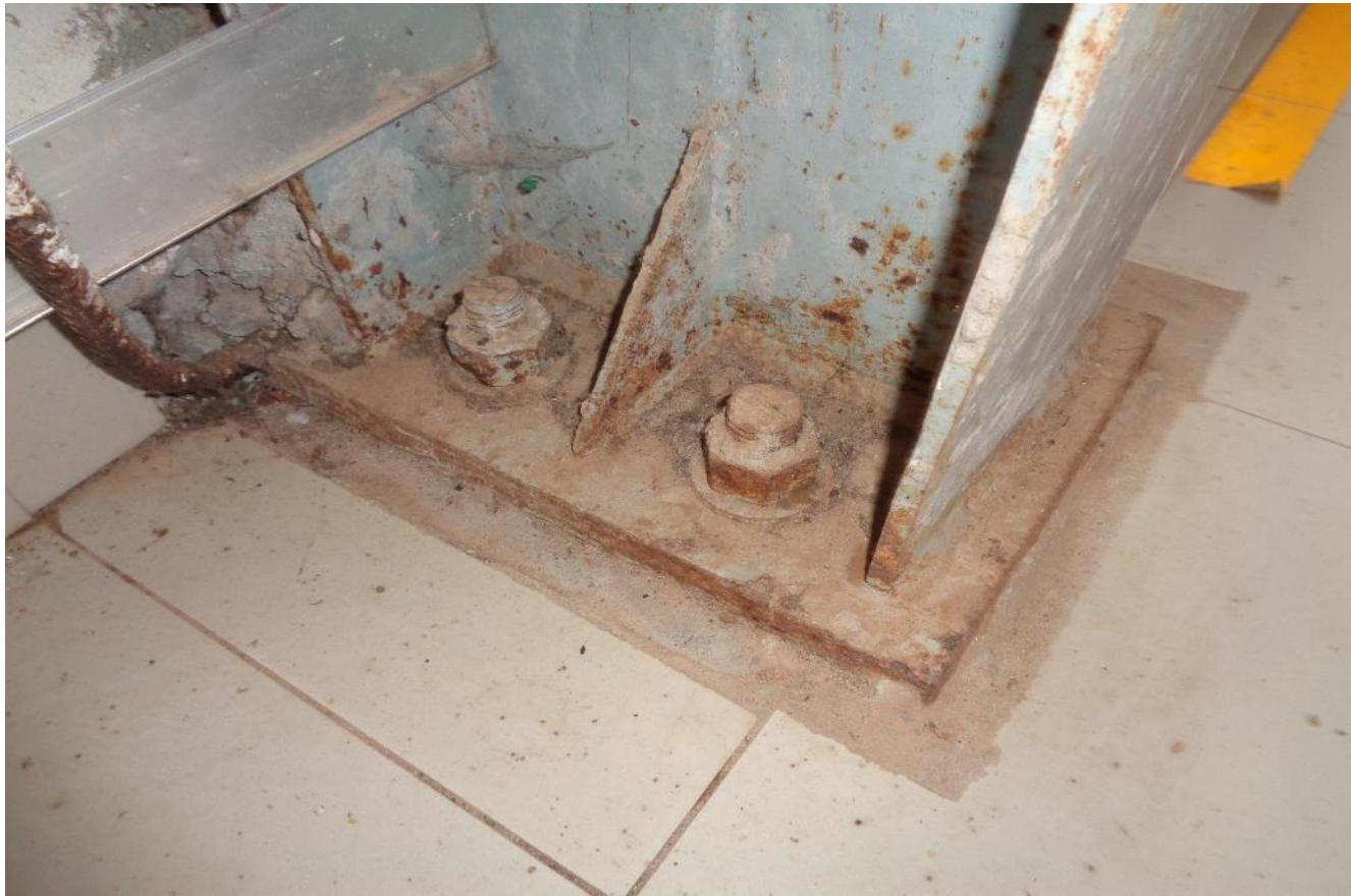
Corrosion found in steel members
