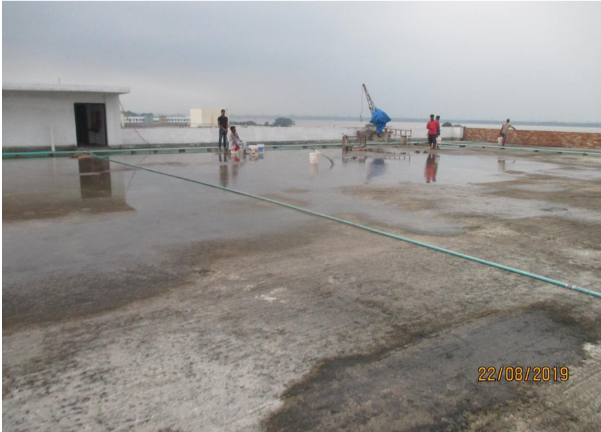
Water ponding was found at roof level.
