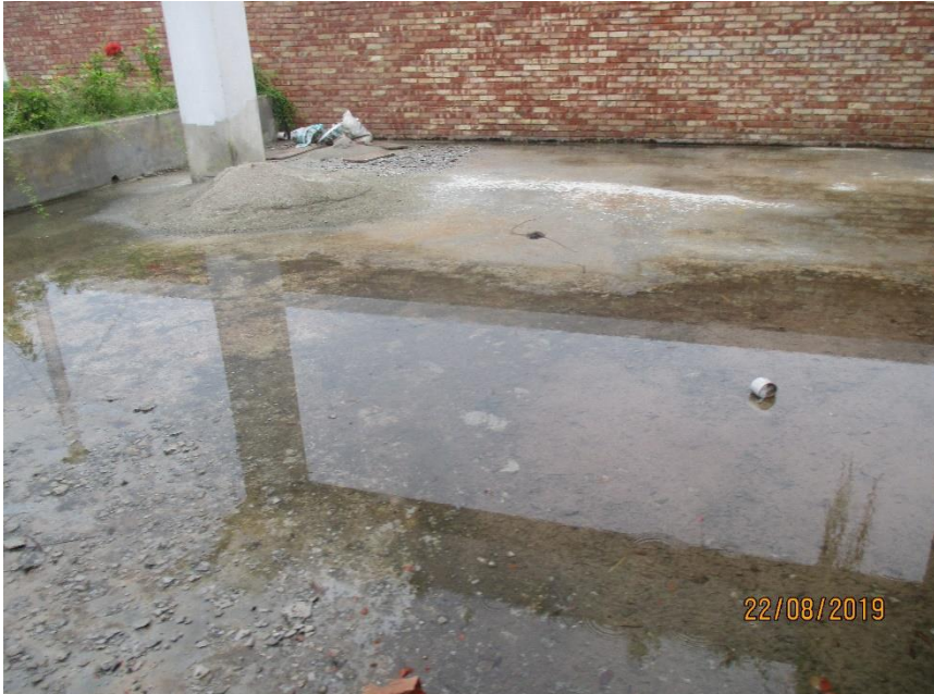
Water ponding was found at roof level.
