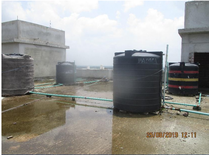
Sign of water clogging
