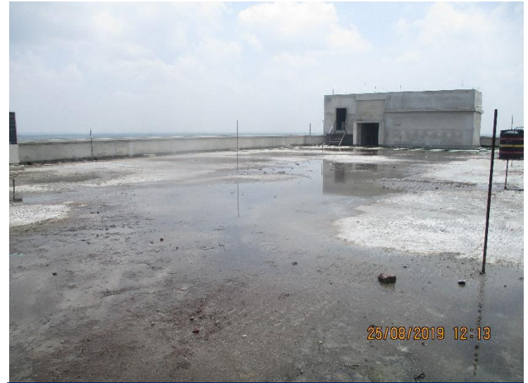
Improper roof drainage system
