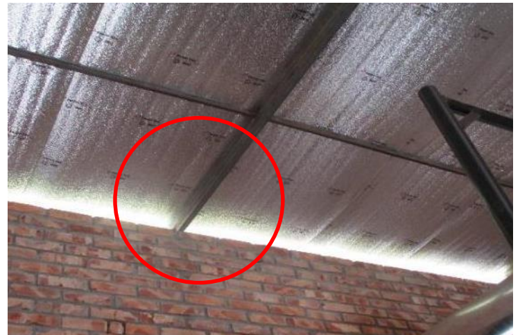
Steel frame rest on masonry wall without adequately anchored.
