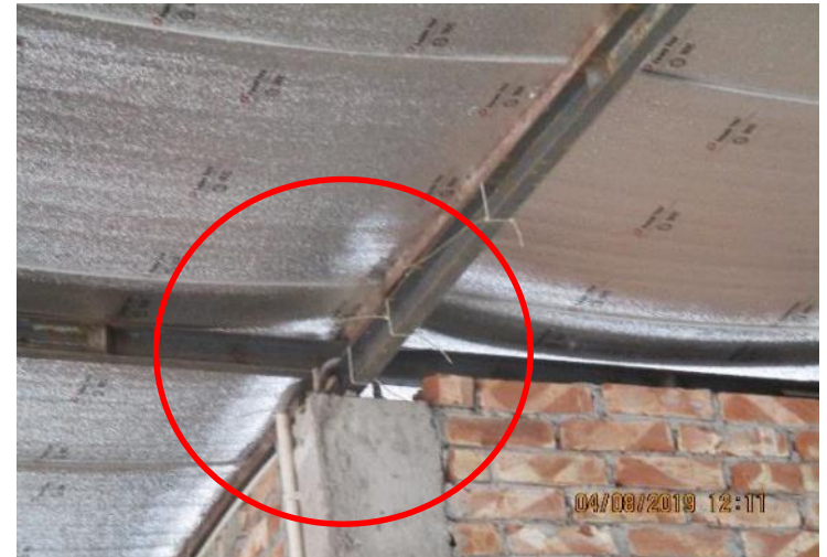
Poor connection details
