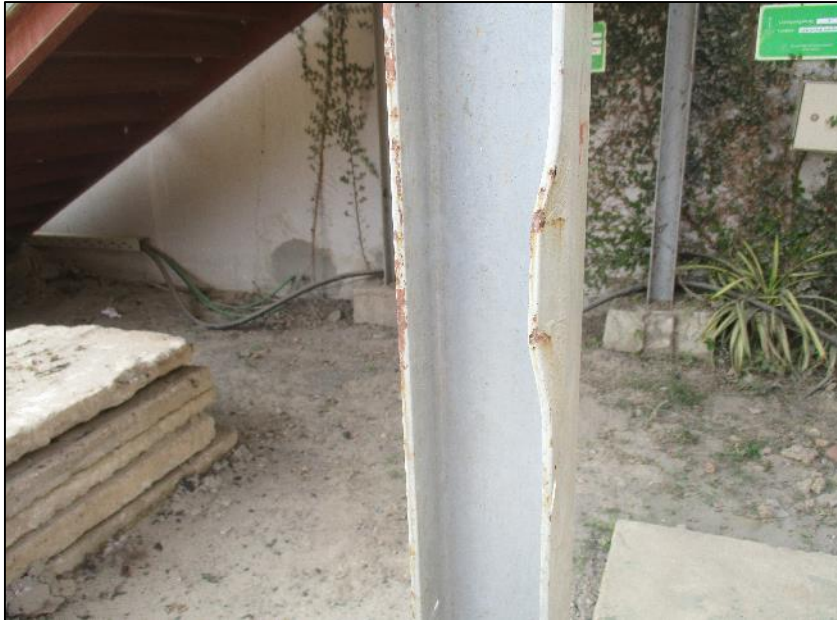
Distorted steel column at external steel stair
