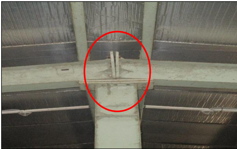
Gap in rafter to rafter connection
