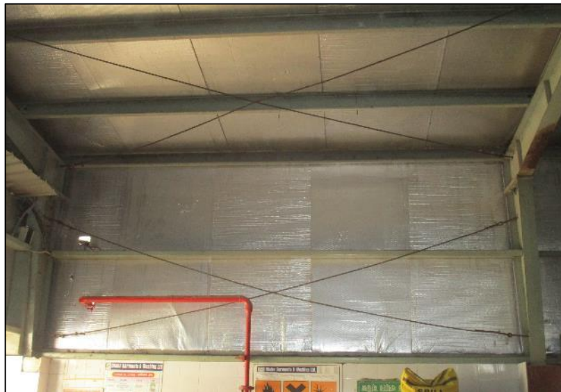
Loose vertical & roof bracing
