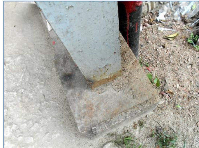
No fixity (pin or fix) between baseplate and short column was observed.
