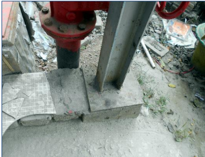
No fixity (pin or fix) between baseplate and short column was observed.
