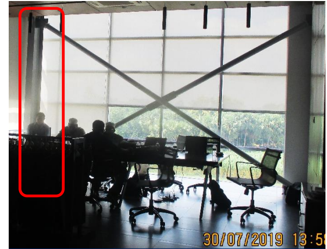
Bracing on 1 st floor missing
