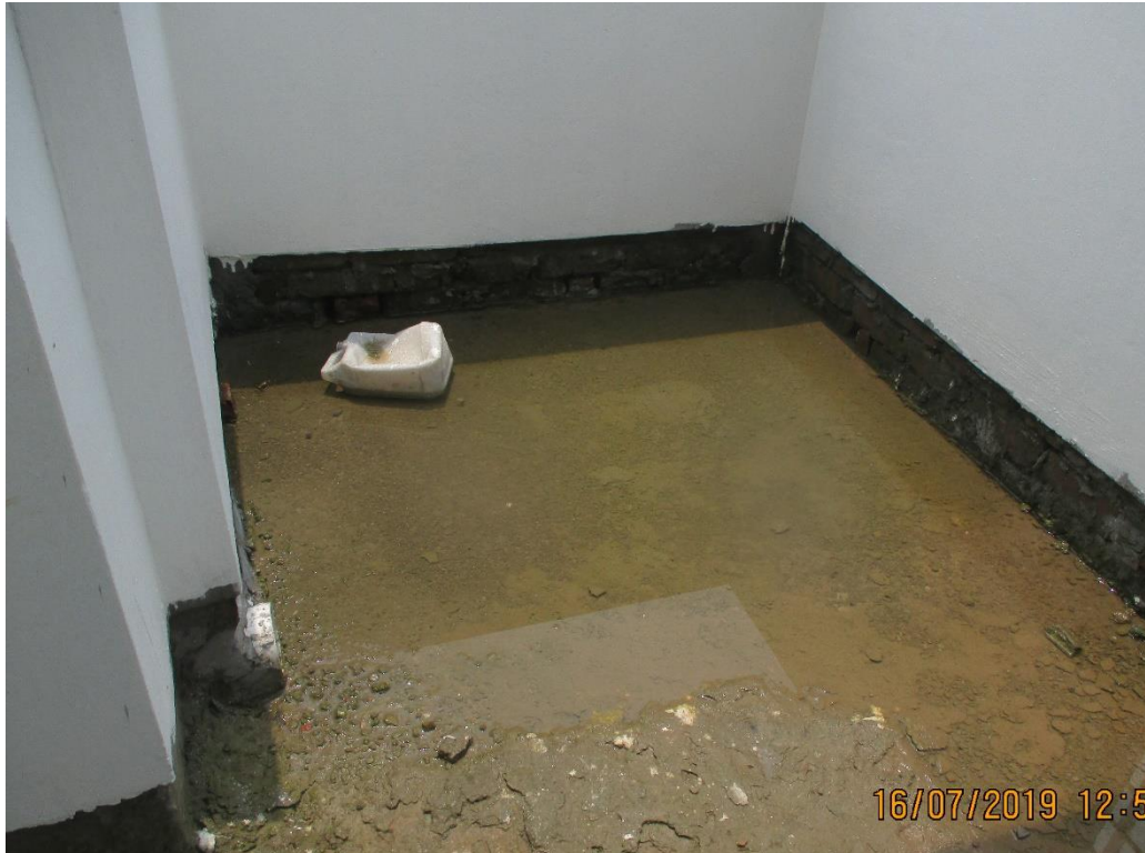
Water ponding observed on 3 rd floor
