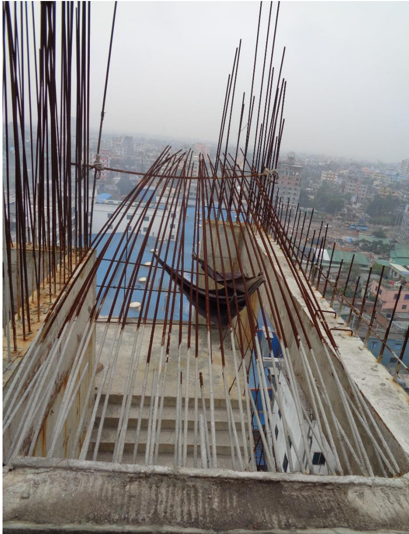
Exposed rebar at Stair
