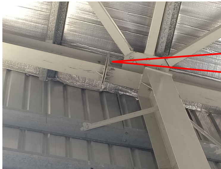
Gap in rafter-rafter joint
