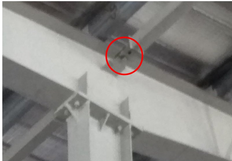
Bolt missing at strut connection
