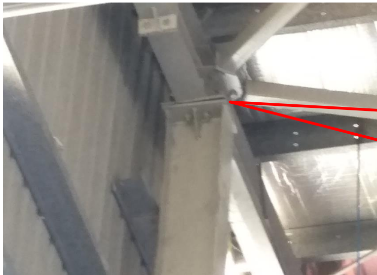
Gap in column-rafter joint
