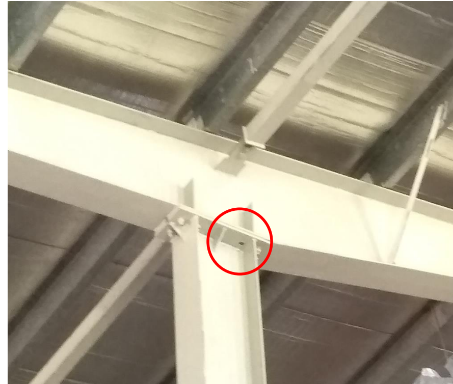
Bolt missing at column-rafter joint
