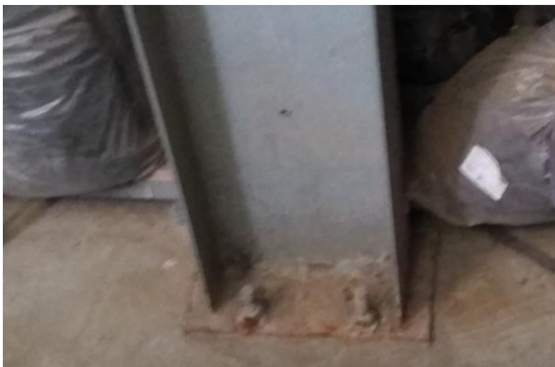
4 nos of bolts were found instead of 6 nos
