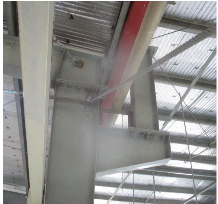
Incomplete separation work of part A & B, Shed-12
