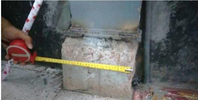
Incomplete retrofitting of short column & base pale, Shed-7
