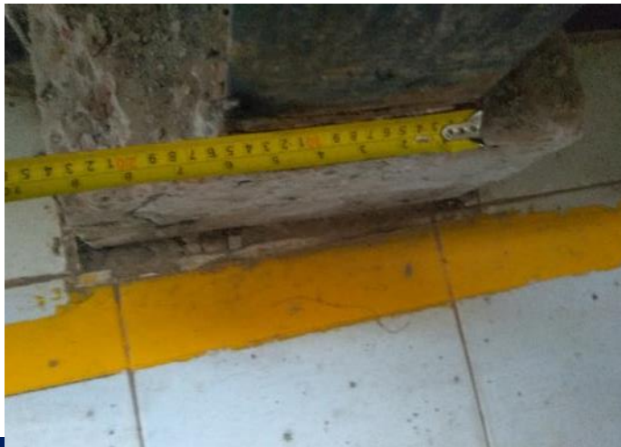
Width of base was measured 150mm instead of 200 mm
