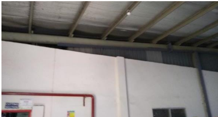
Incomplete retrofitting of short column, base pale, column & rafter, Shed-10
