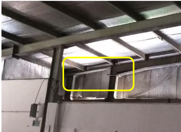
No rafter in marked location
