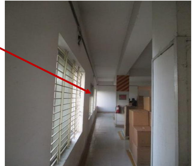
2.1m wide cantilever on East side which was not shown in drawing
