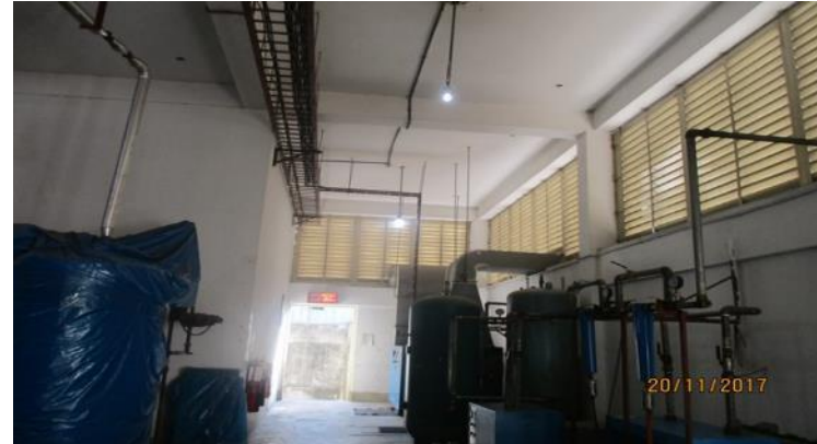
Inside Boiler & Pumphouse Building
