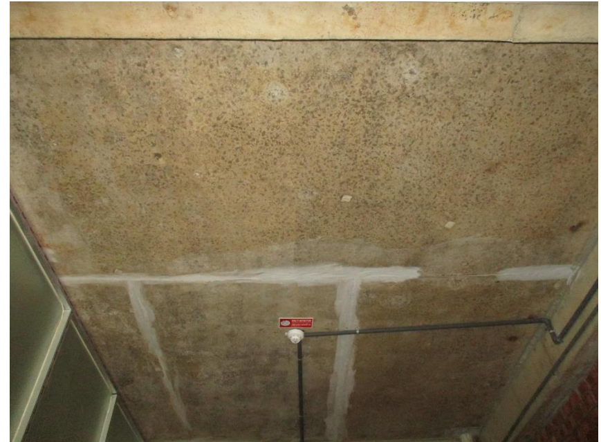
Sign of dampness underside the down slab.
