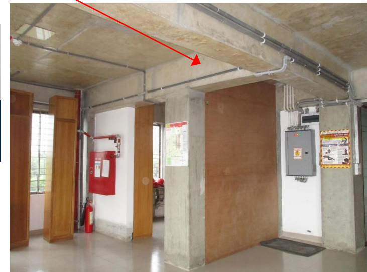
Beam at 2 nd floor not match with dwg.
