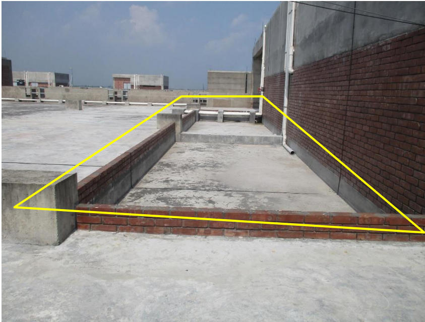
Down area on the roof.
