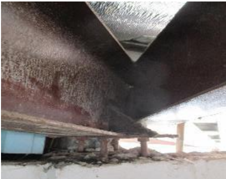
Gap in RC column-steel rafter connection
