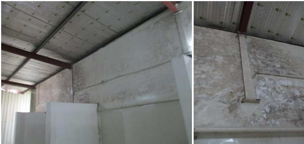
Dampness on peripheral wall
