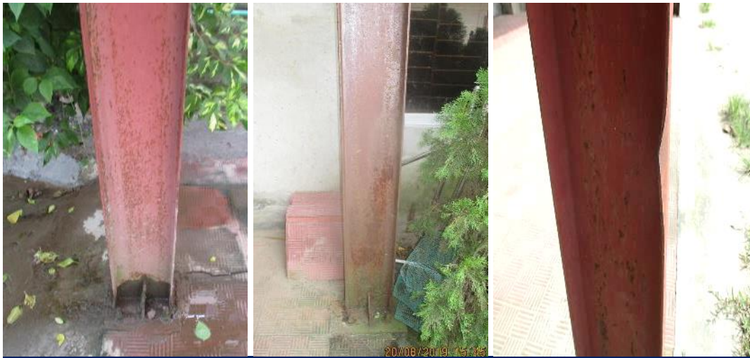
Corrosion in steel column
