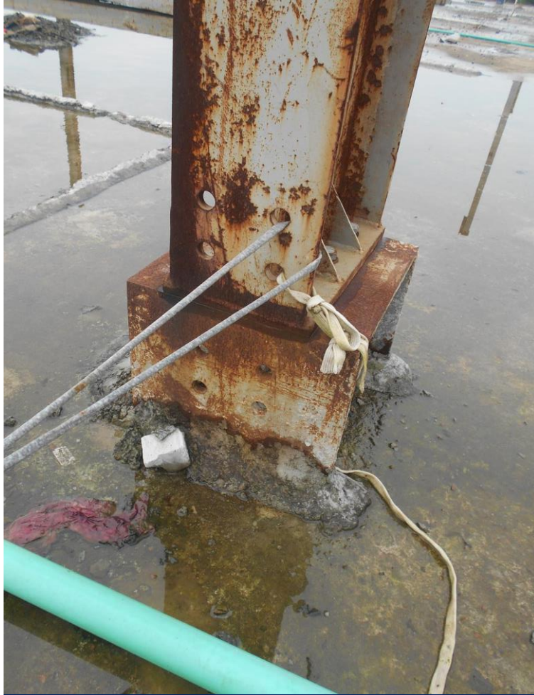
Corrosion in steel column
