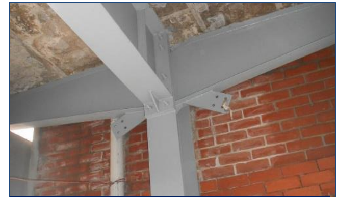
Bracing not installed on site
