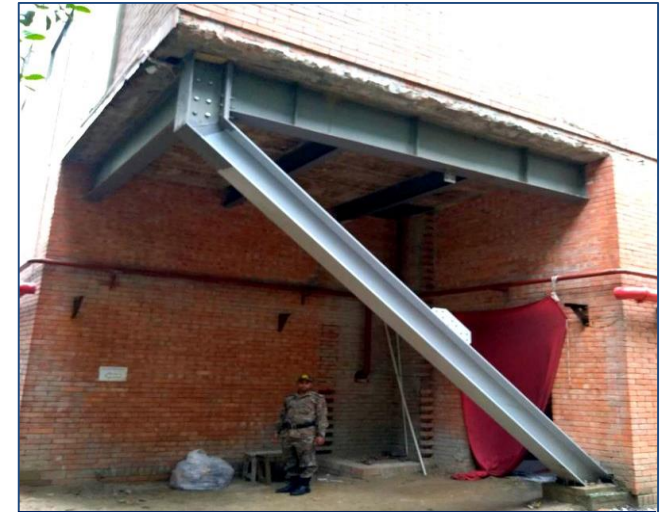
Bracing not installed on site
