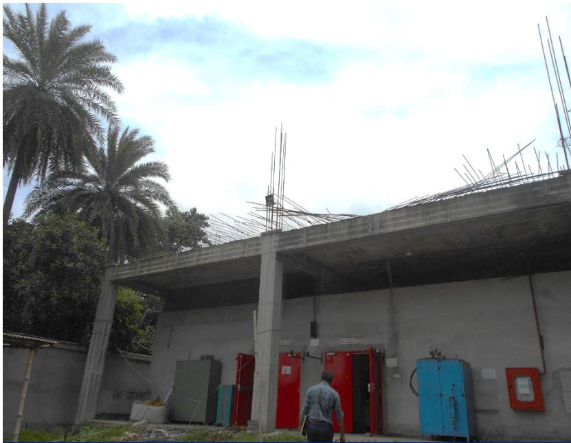
Exposed Rebar at south
