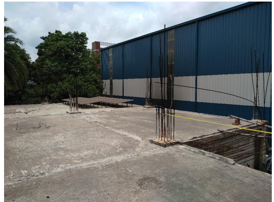
Exposed Rebar on roof
