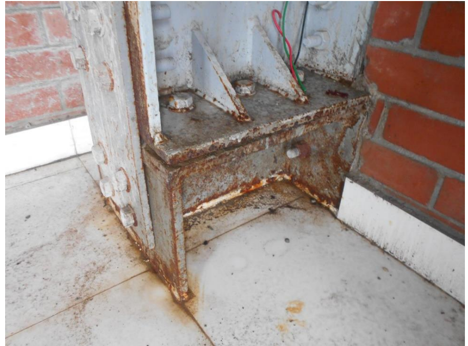
Corrosion at column joint
