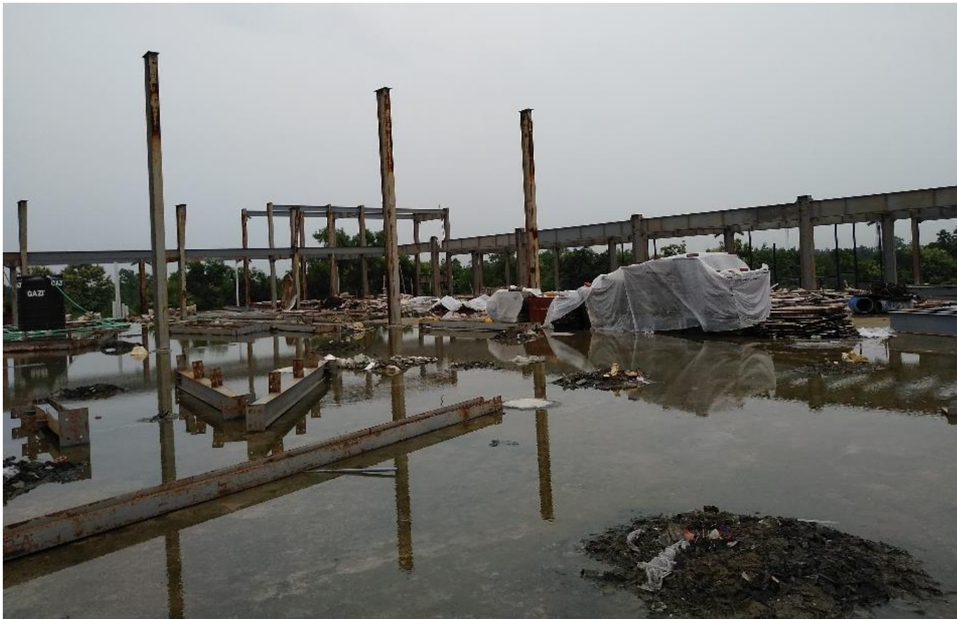
Construction debris on the 2 nd floor roof.
