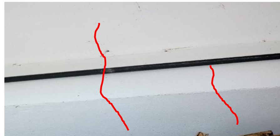
Cracks on peripheral beams
