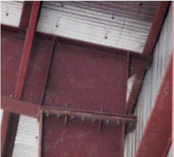
Gap between column-rafter connection
