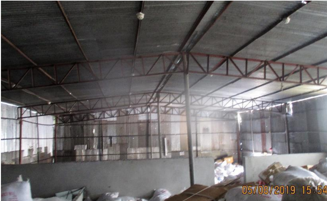
Missing load transfer in long direction
