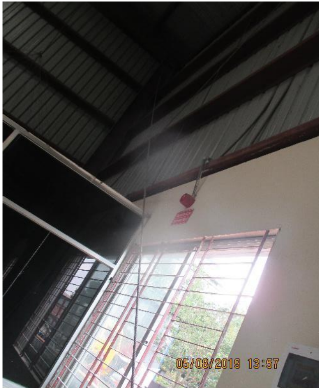
Loose vertical bracing
