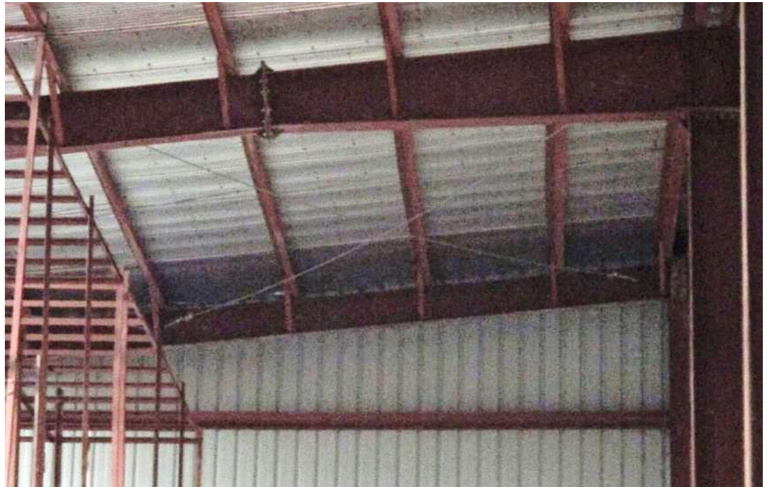
Loose roof bracing
