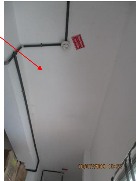
Cantilever slab with cracks
