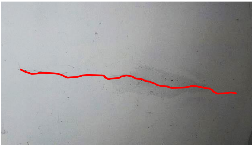
Water ingress through cracks on slab
