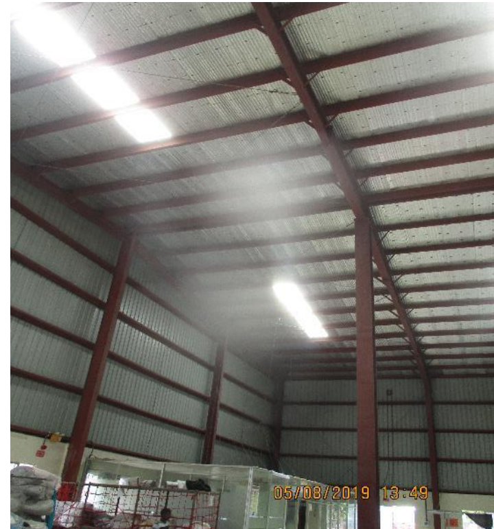
Loose roof bracing
