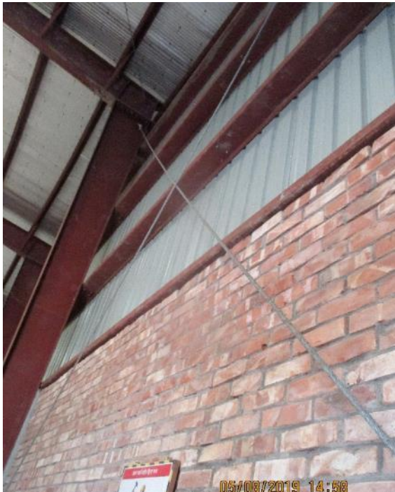
Loose vertical bracing
