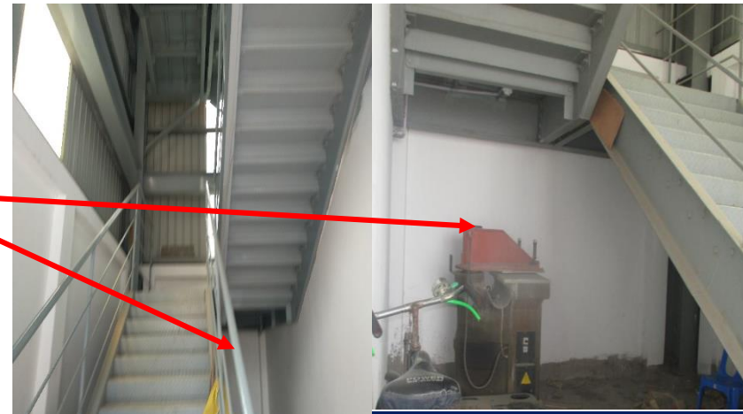
No Bracing at GF level
