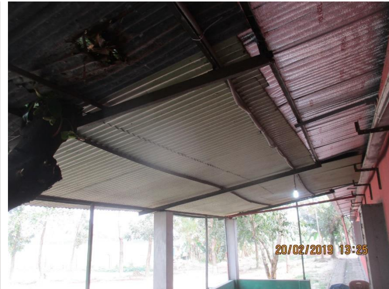
Flimsy steel roof frame
