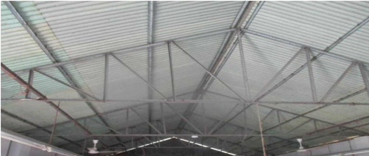
Internal truss system with no roof bracing or vertical bracing
