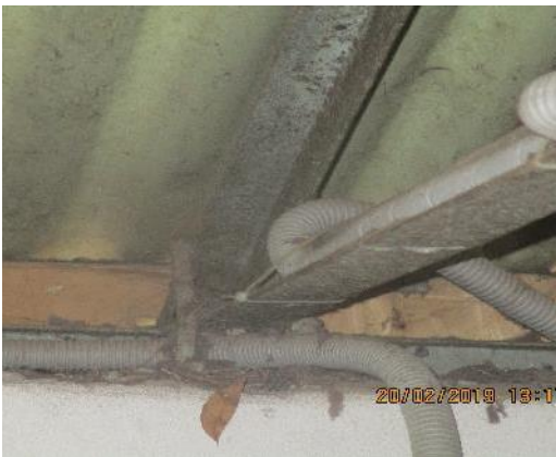
Poor welding joint at end point
