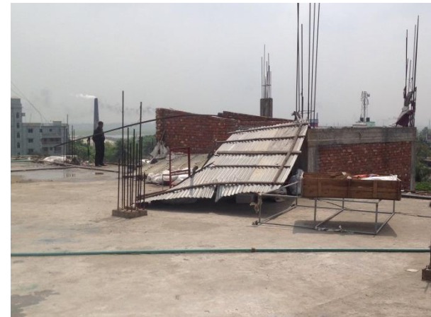
Apparently loose metal sheeting at Roof level
