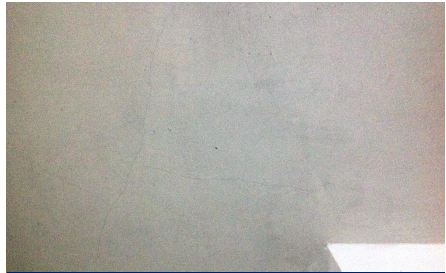
Cracking to underside of flat slab adjacent to column
