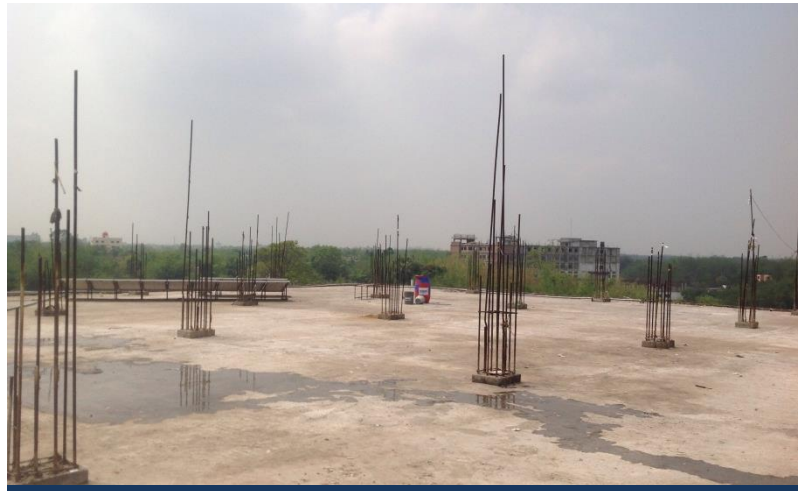
Lack of Fall Barrier to Roof
