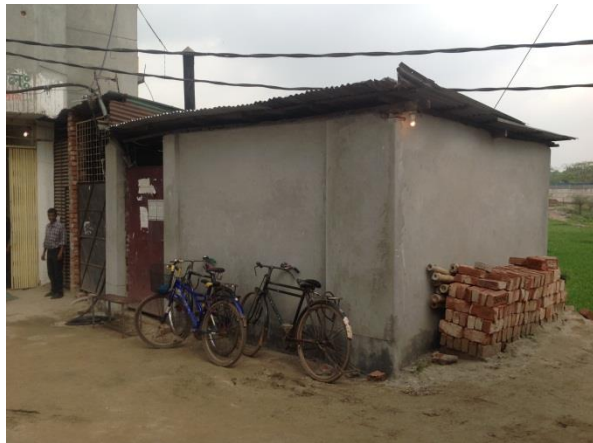
Lightweight Steel Roof to Ground Floor Generator Room
