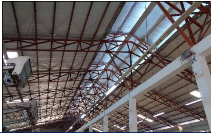
Steel Column Rafter system
