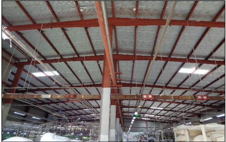
Steel Column Rafter system
