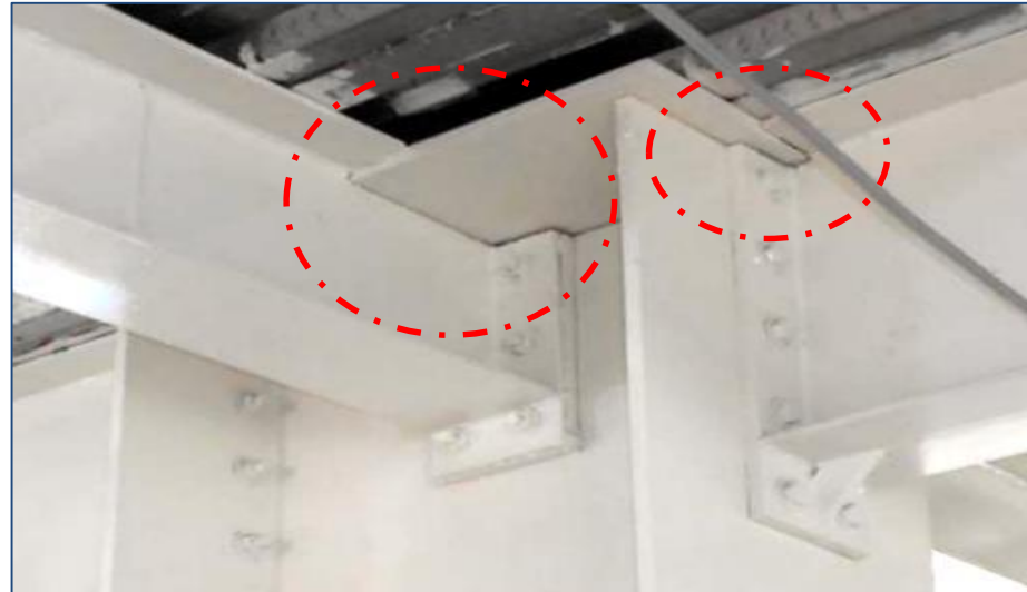
Top flange found cut near the joint
