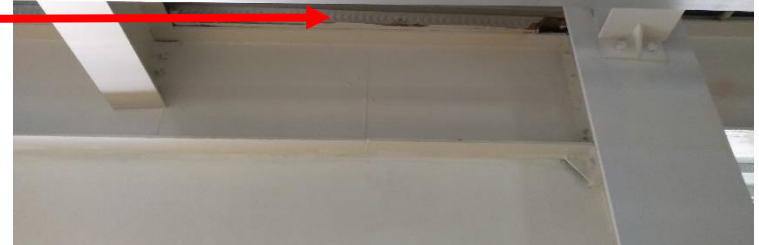
Deflected portion of deck slab
