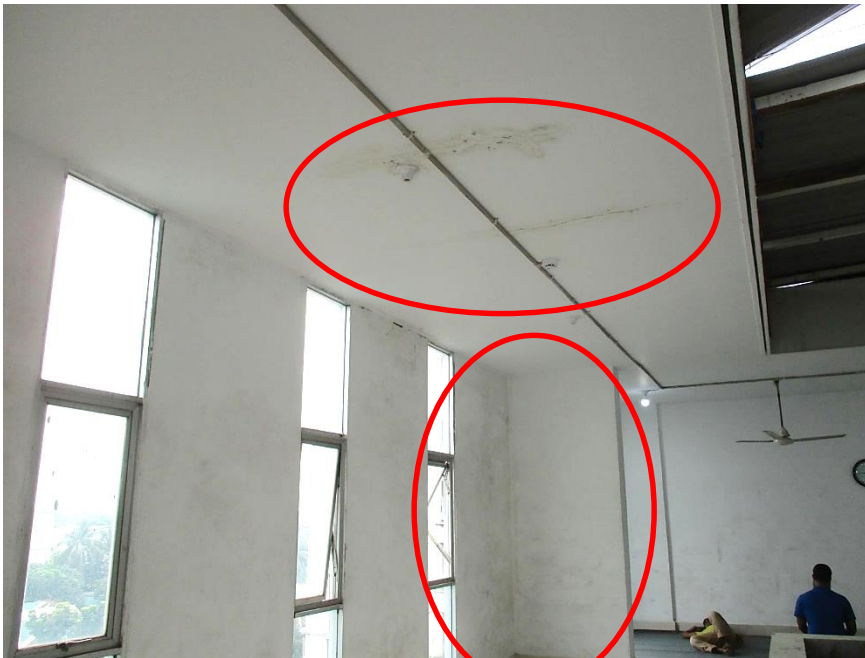
Sign of water damage of Medical Building.
