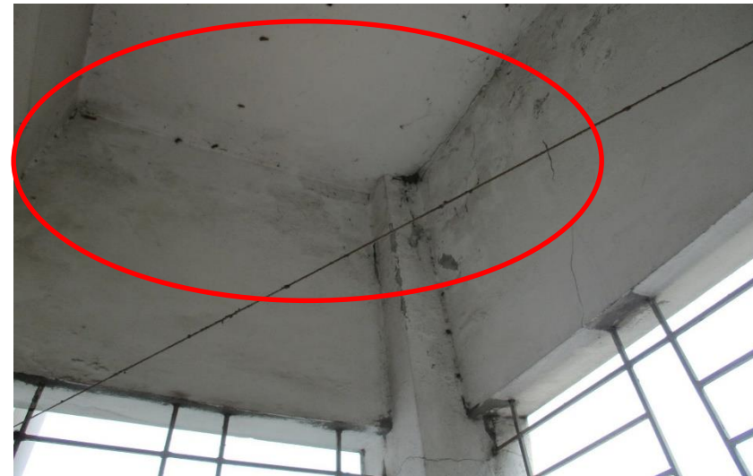
Water ponding was observed on the roof and dampness was observed on wall. Building engineer to apply proper repair method.
