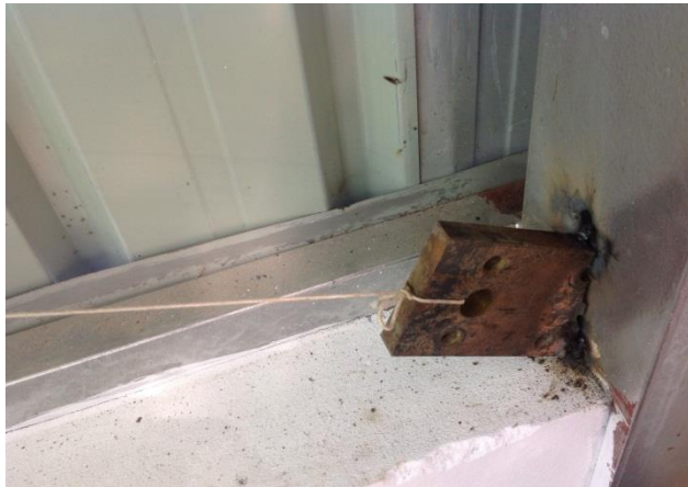
Bracing details not evident in several locations – Engineer to review
