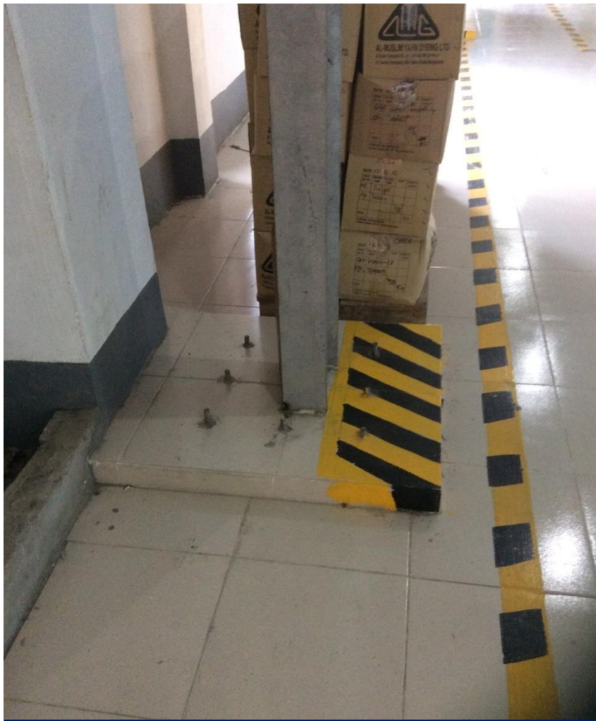
Steel columns connected to First floor slab. Engineer to confirm capacity of slab to take additional loading.
