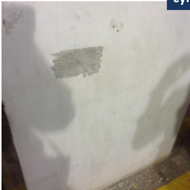
Tested Basement level Column – Stone Chips
