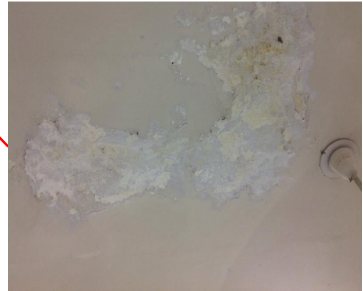
Water ingress to Slab- 2 nd floor
