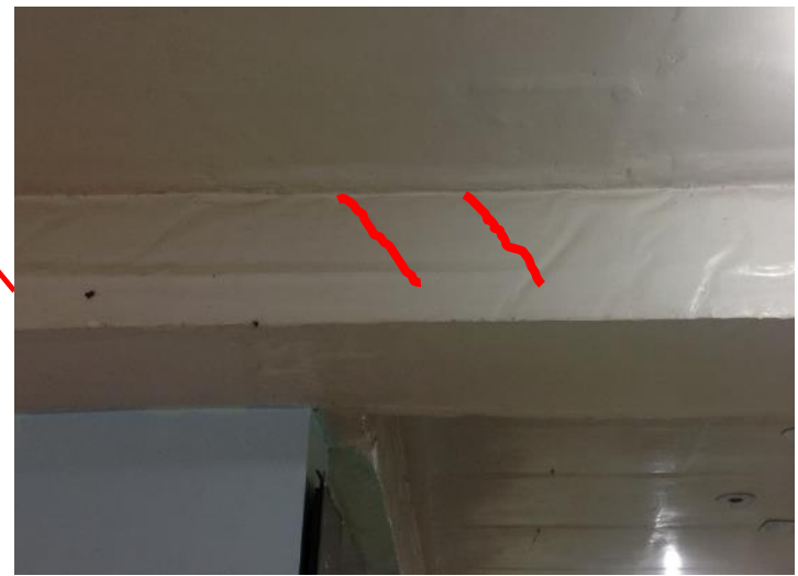
Beam Cracking – 1 st Floor Accessories Backup Store
