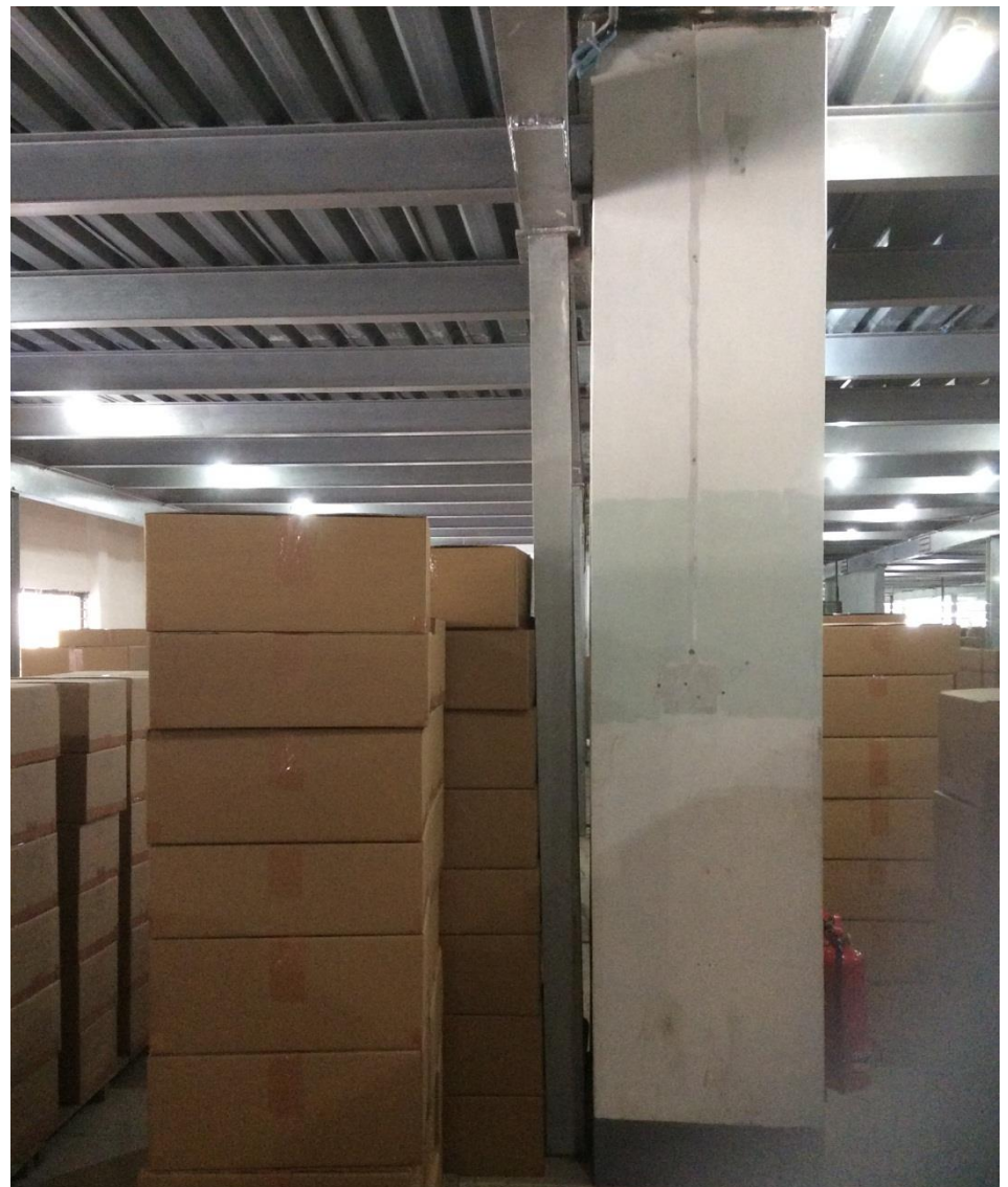
Steel columns out of plumb. Engineer to confirm Stability of structure.
