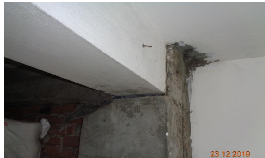
Improper connection with existing beam
