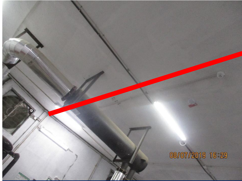
Floor beam missing
