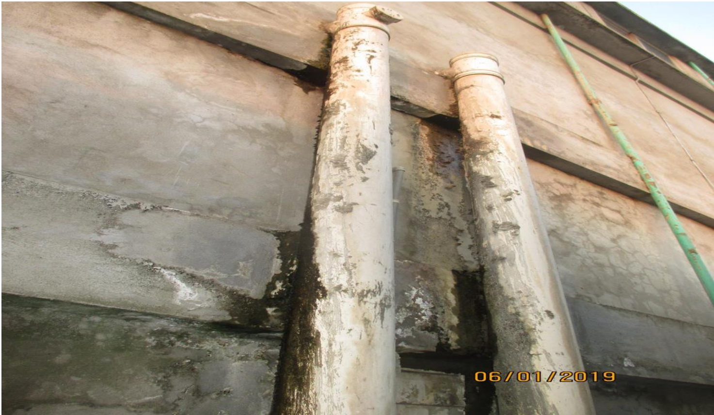
Water intrusion in exterior façade from sanitary pipe.
