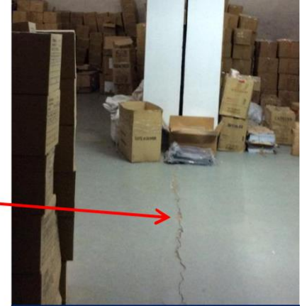
Cracks in Ground floor slab
