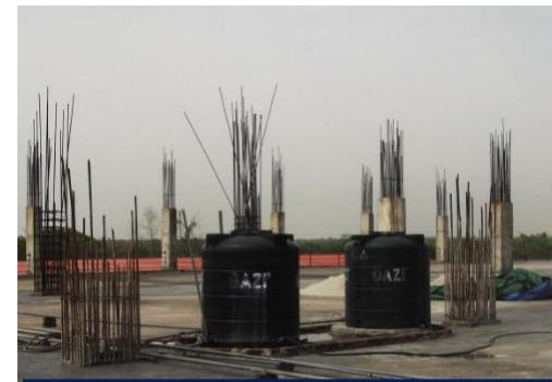
Water tanks loads
