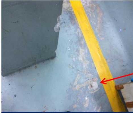
Cracks in 1 st floor slab
