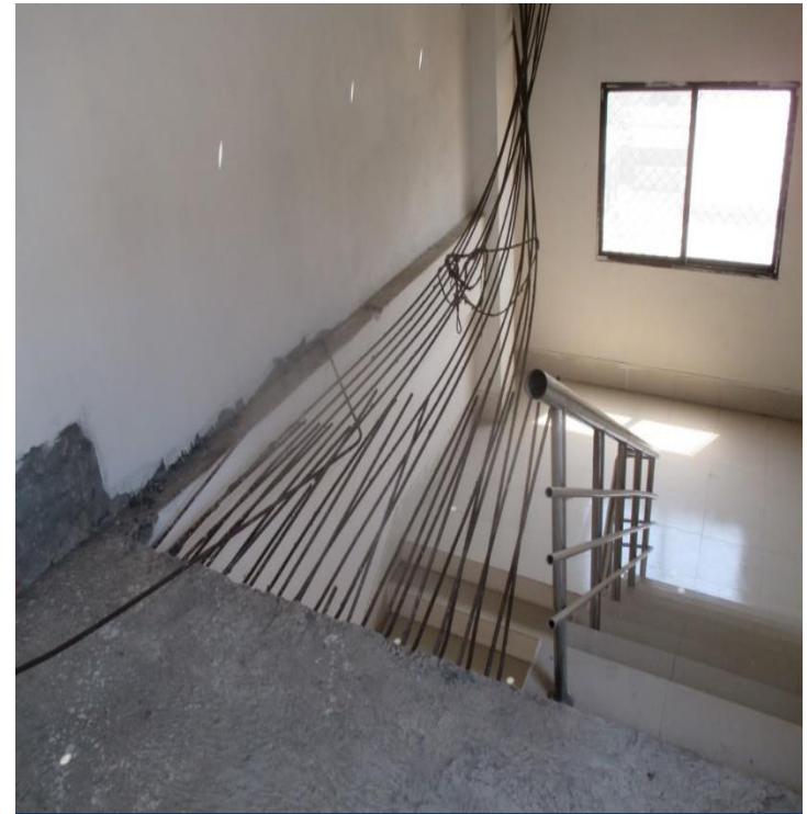
Reinforcement of Stair slab were found exposed
