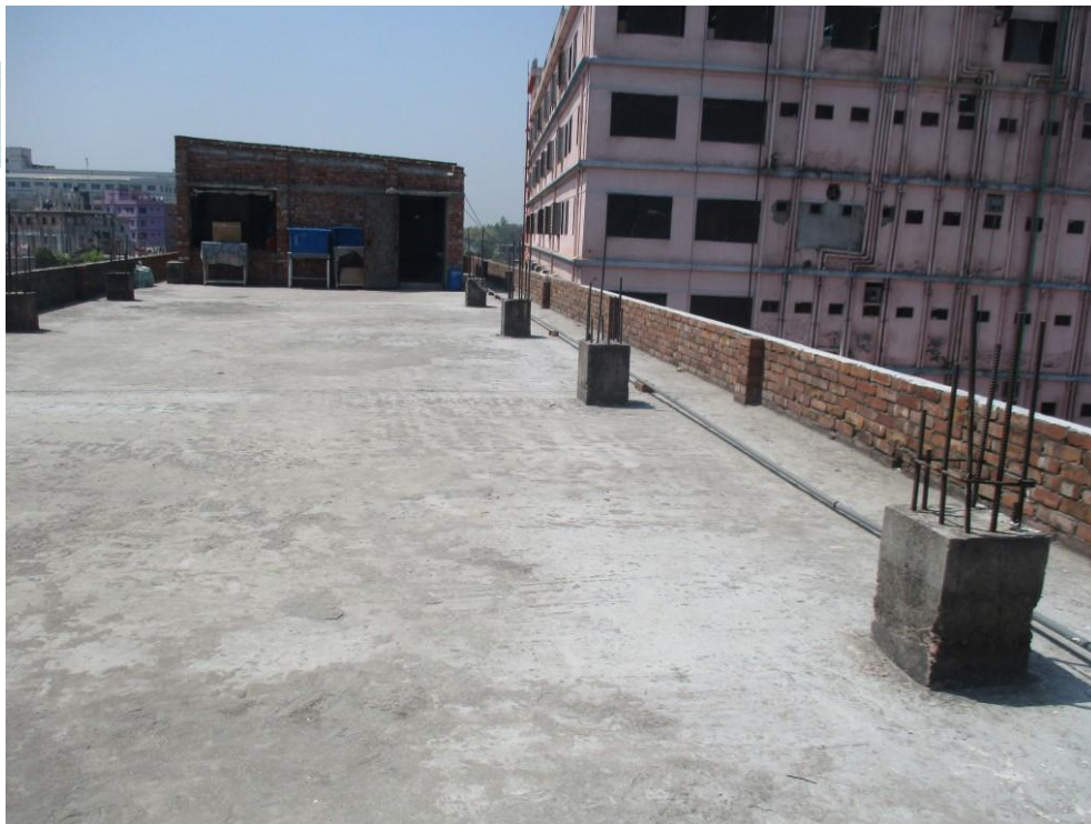
Reinforcement of columns were found exposed on existing roof top
