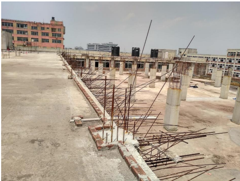
Expose rebar at roof
