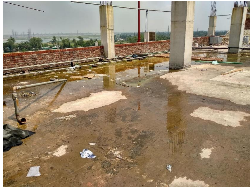
Improper roof drainage system
