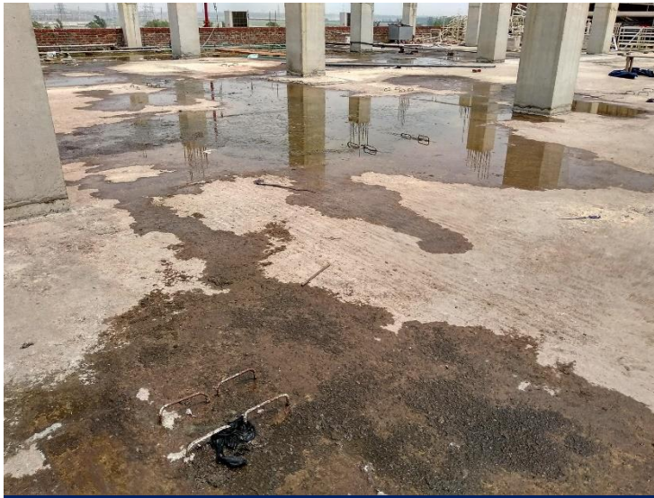
Lack of water proofing layer
