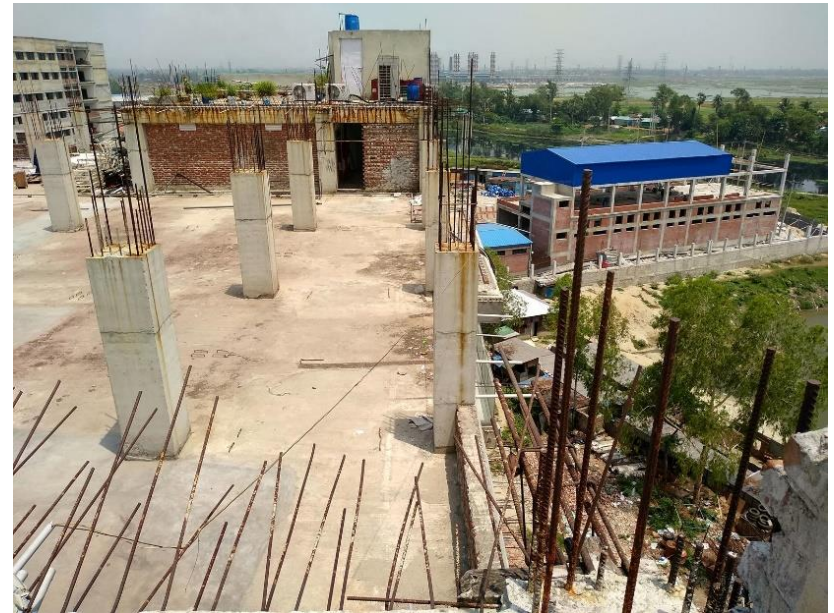
Exposed rebar at Column
