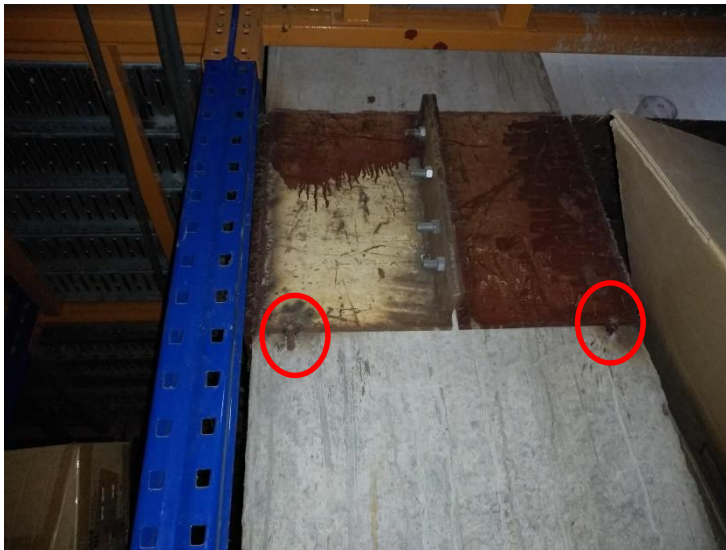
Steel plate with inadequate anchorage
