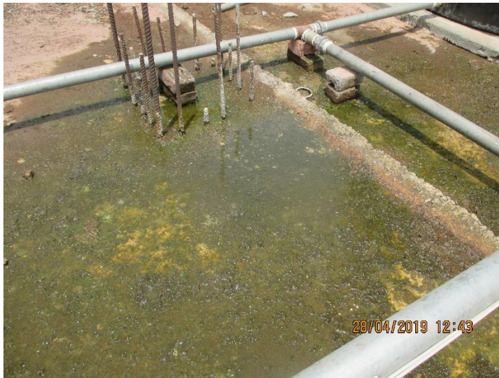
Sign of water clogging
