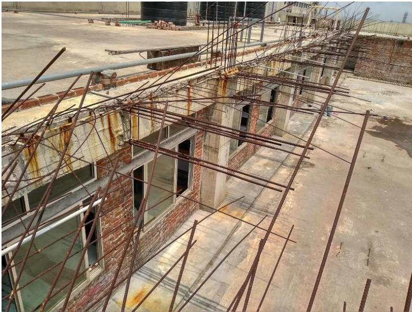
Exposed rebar at Beam & Slab
