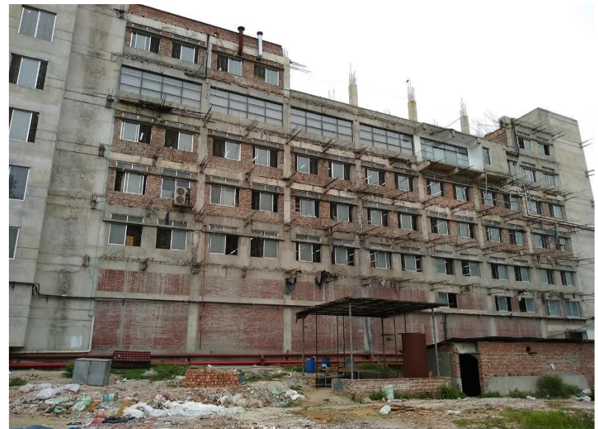
Expose rebar at South
