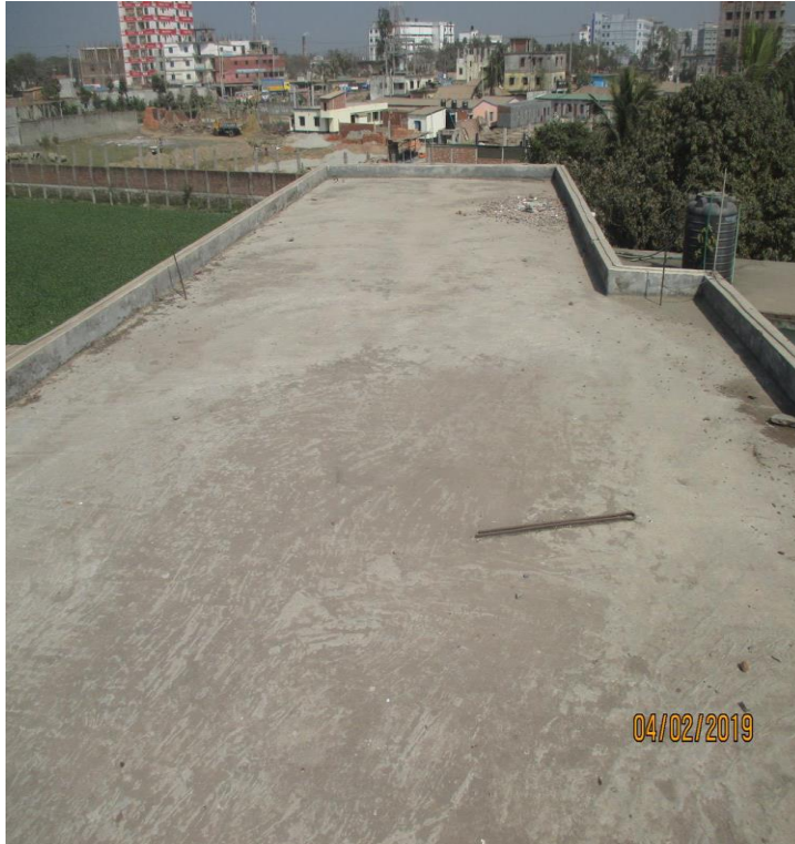
Signage of water ponding was found at roof level
