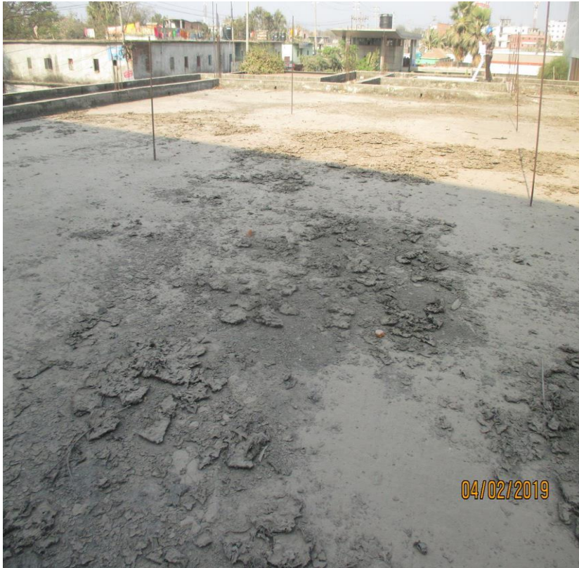
Signage of water ponding was found at roof level
