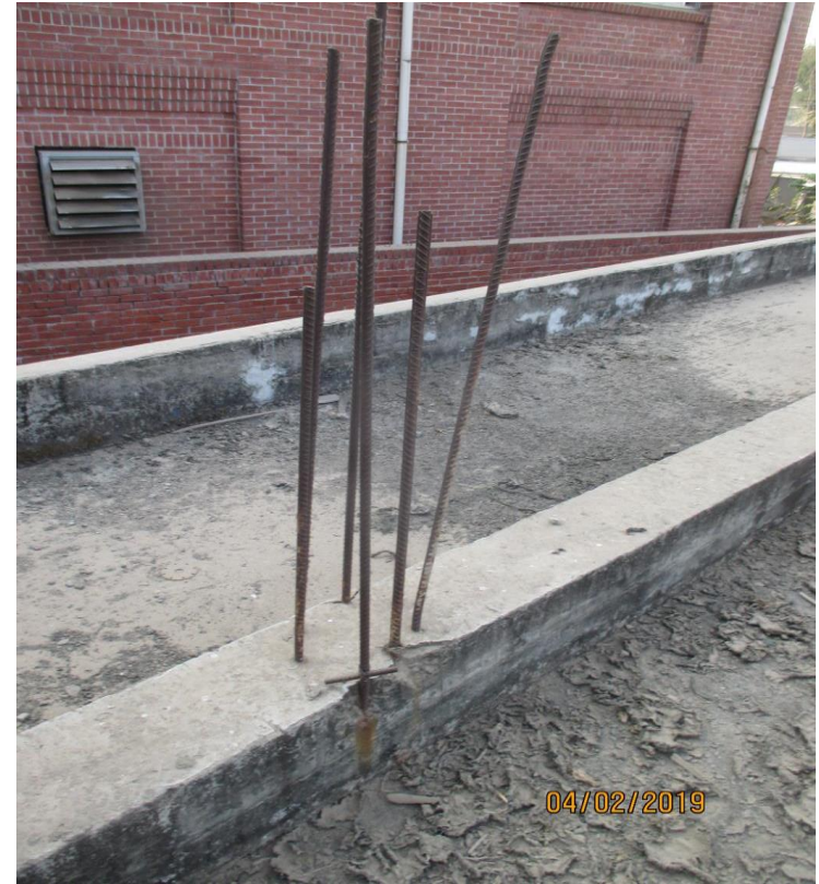
Column re-bar was found exposed at roof level
