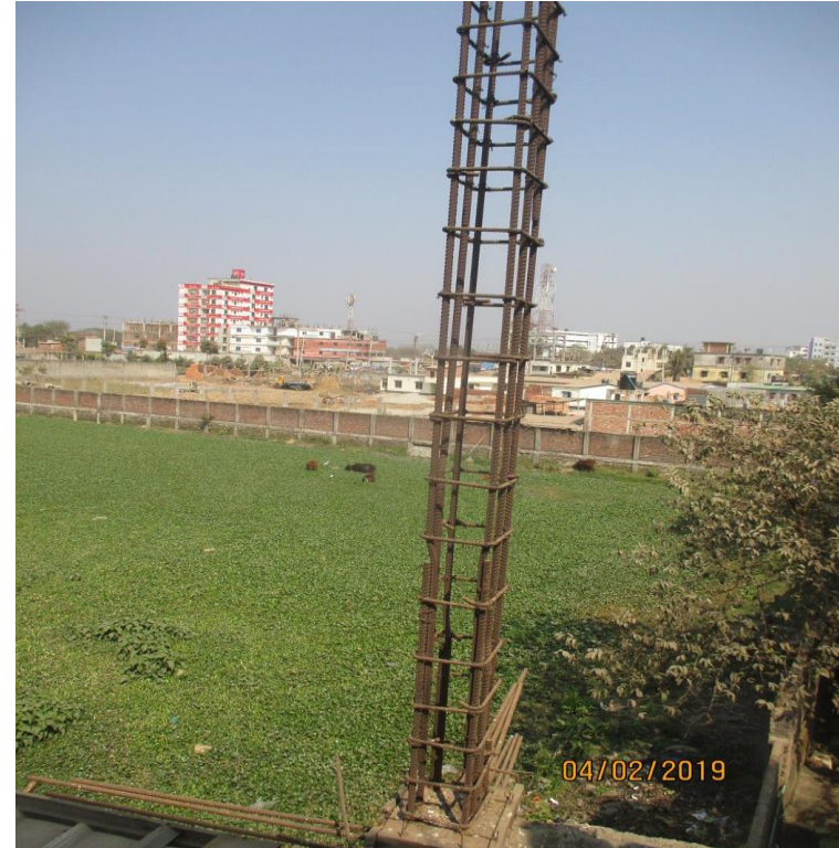
Column re-bar was found exposed at roof level
