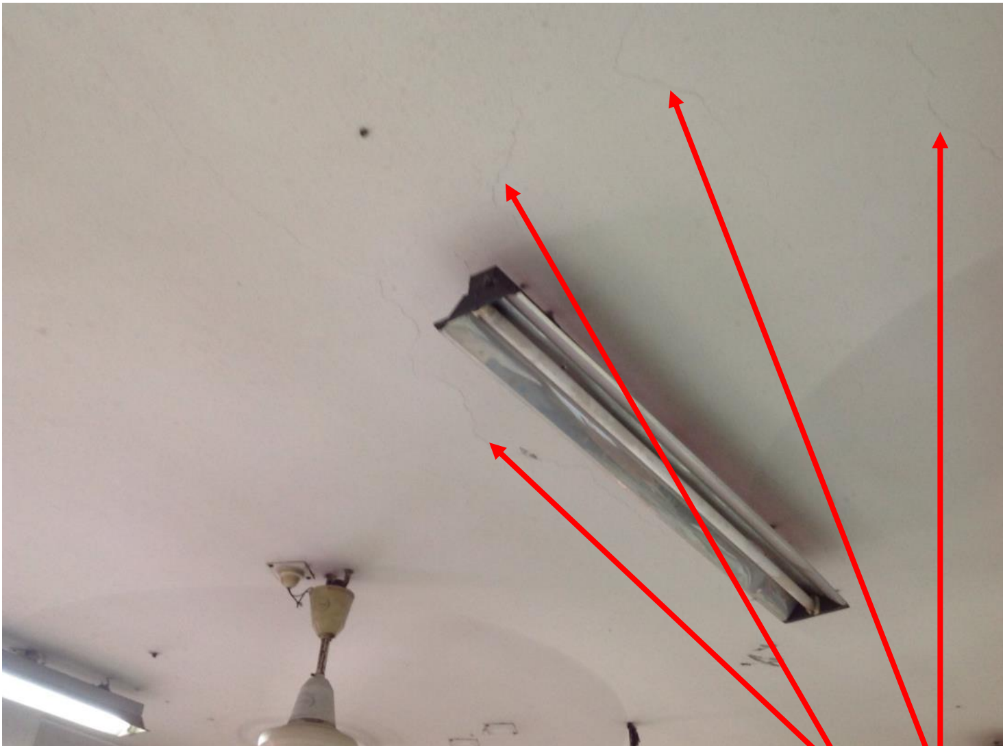
Minor cracking to underside of slab
