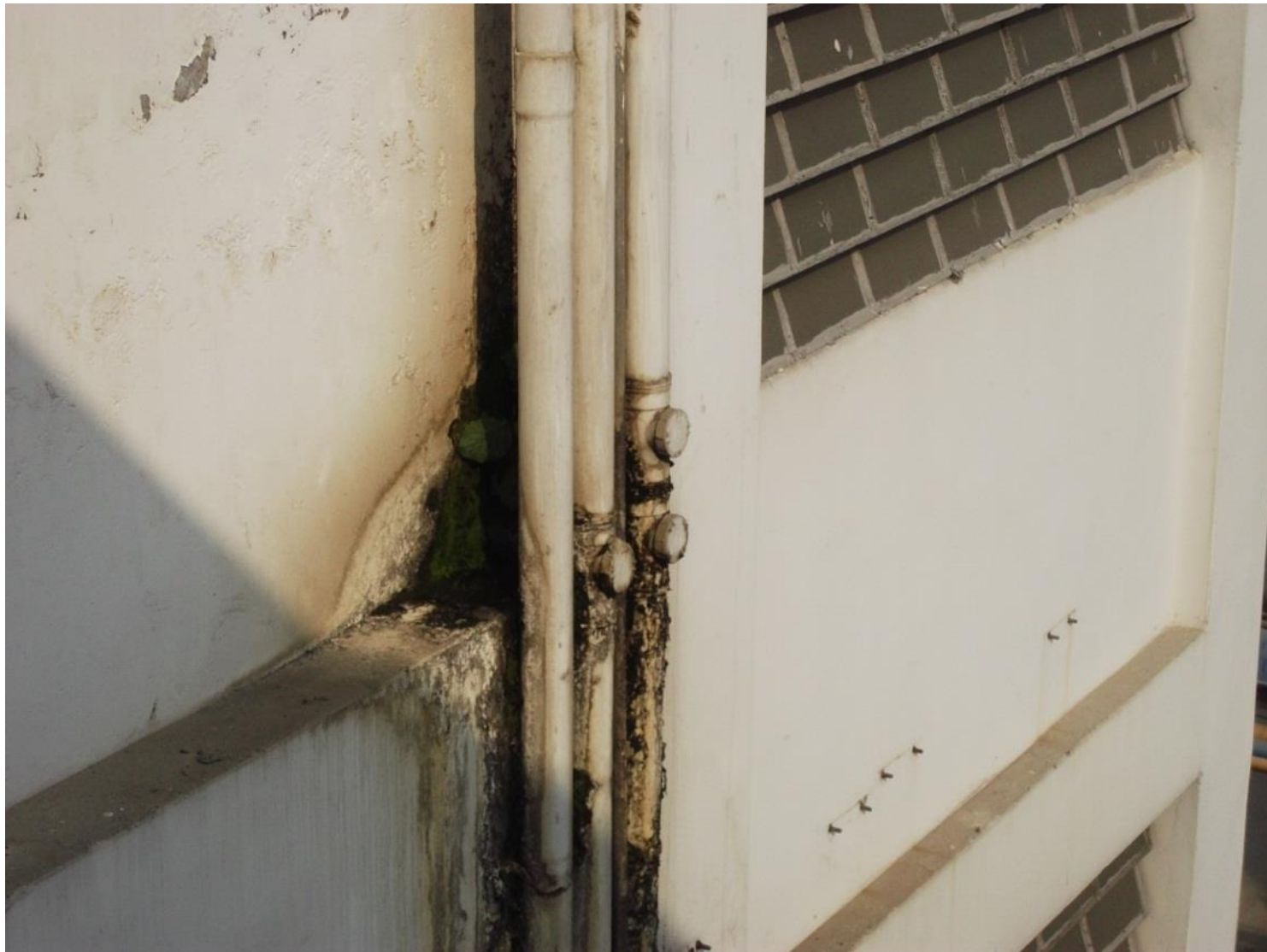
South Elevation – Maintenance Required
