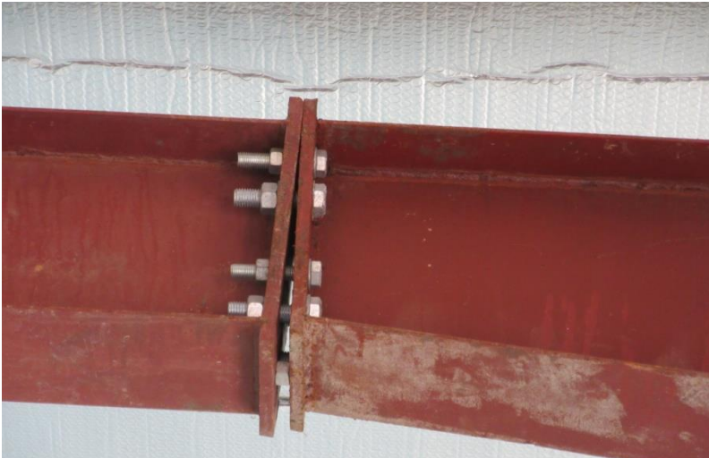
Apparently not a full contact of the connection plates.
