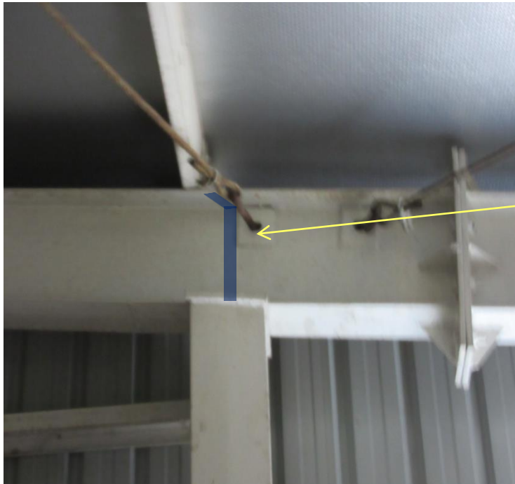
Missing steel rib for the transfer of the vertical load to the column
