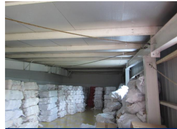
Apparently some of the bracing are tied very loosely
