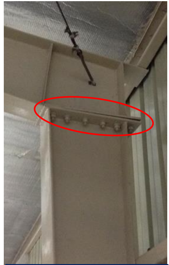
Building 2 – Roof beam/column connection – gap between endplates
