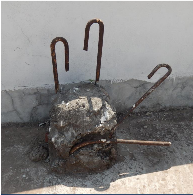
Evidence of low yield strength bars on roof
