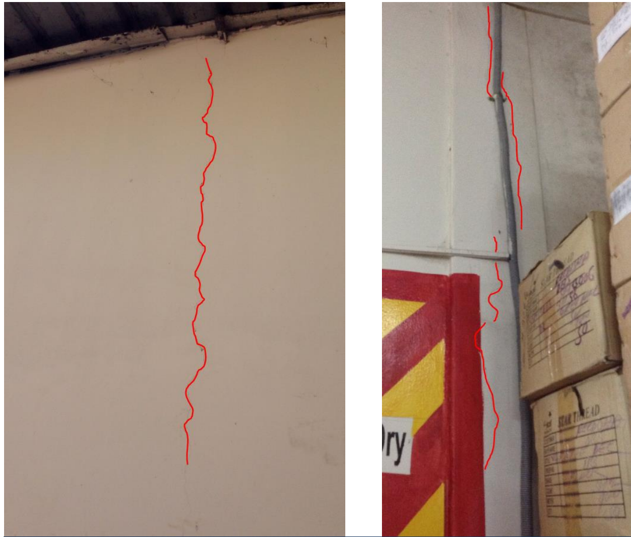
Cracking noted in wall where steel columns are embedded.
