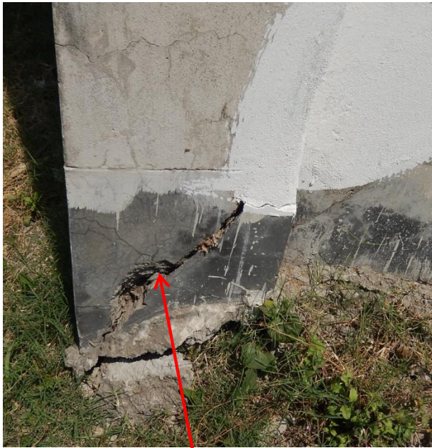
Cracking in base of column/foundation caused by / or worsened by vegetation growth
