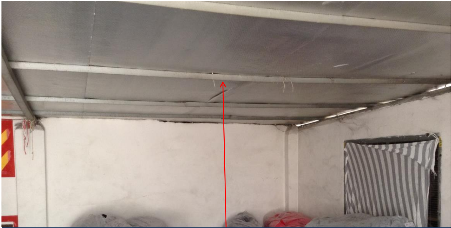
L-purlins appear not adequate to resist high wind loads
