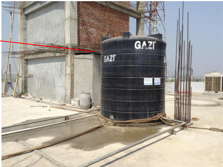
• 10,000 litre Gazi water tank
