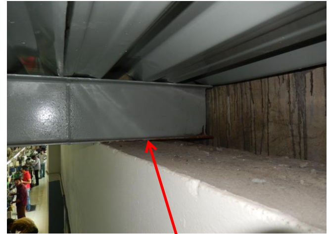
No anchorage detected between roof deck and concrete beams
