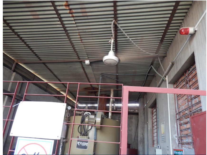
Metal deck in boiler building
