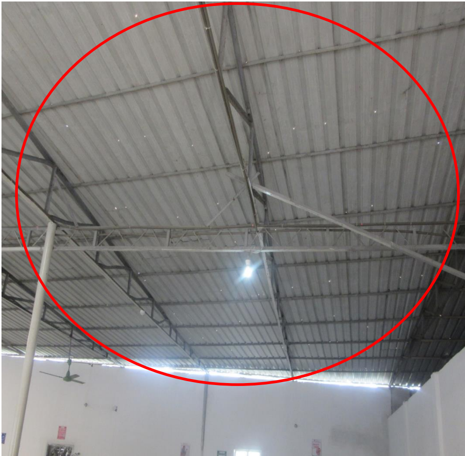
No roof bracing in Dining Shed
