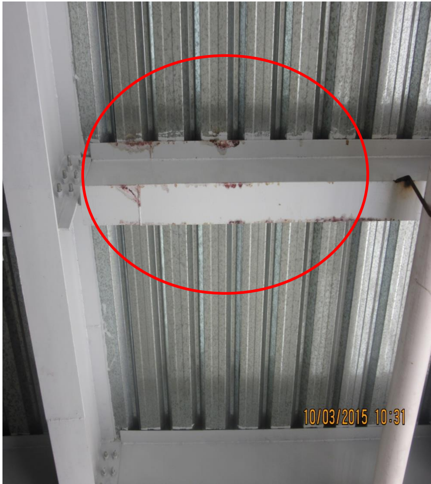
Corrosion of the steelwork commencing under the concrete roof section of Main Building
