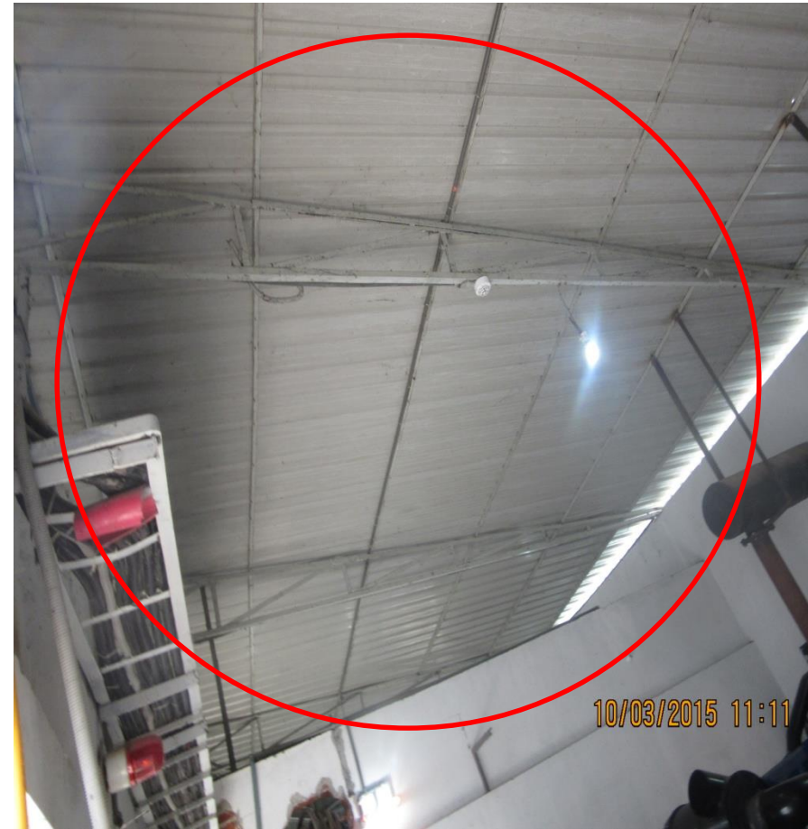
No roof bracing in Generator/Sub-station room
