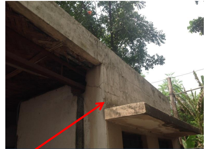
Cracking to walls of Building 2
