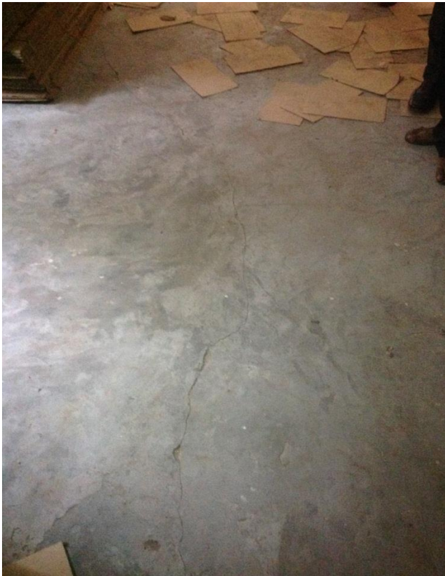
Building 3 cracking to ground floor slab
