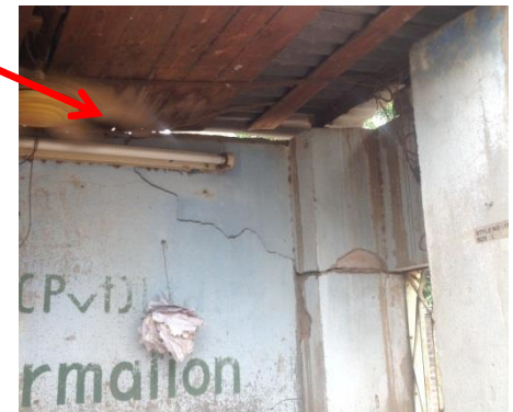
Cracking to wall and brick column in Guard House
