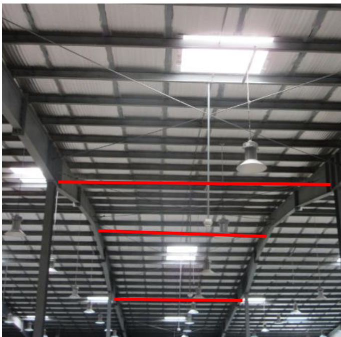
Roof bracing – no obvious compression struts
