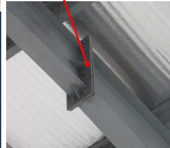
Roof girder connection appears to have rotated
