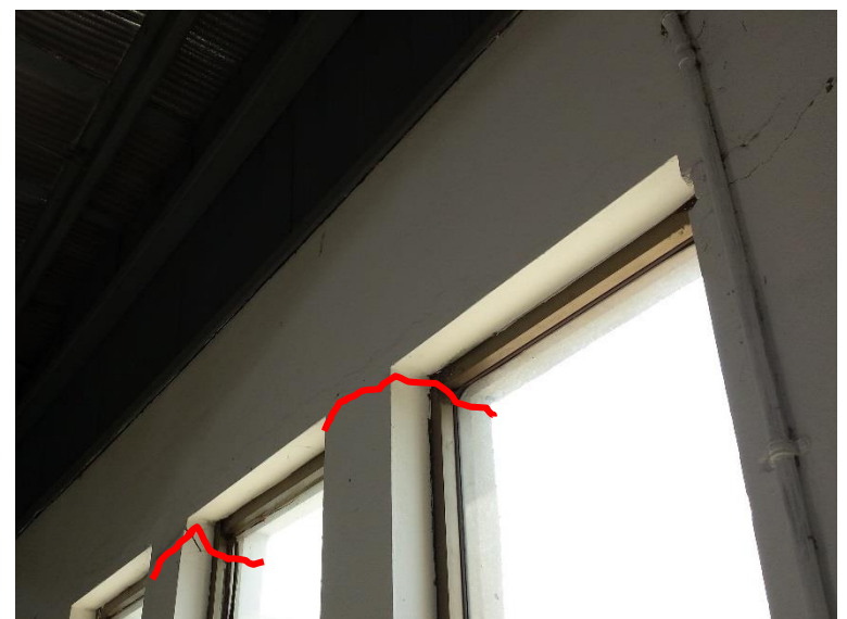
Fully cracked window pillars
