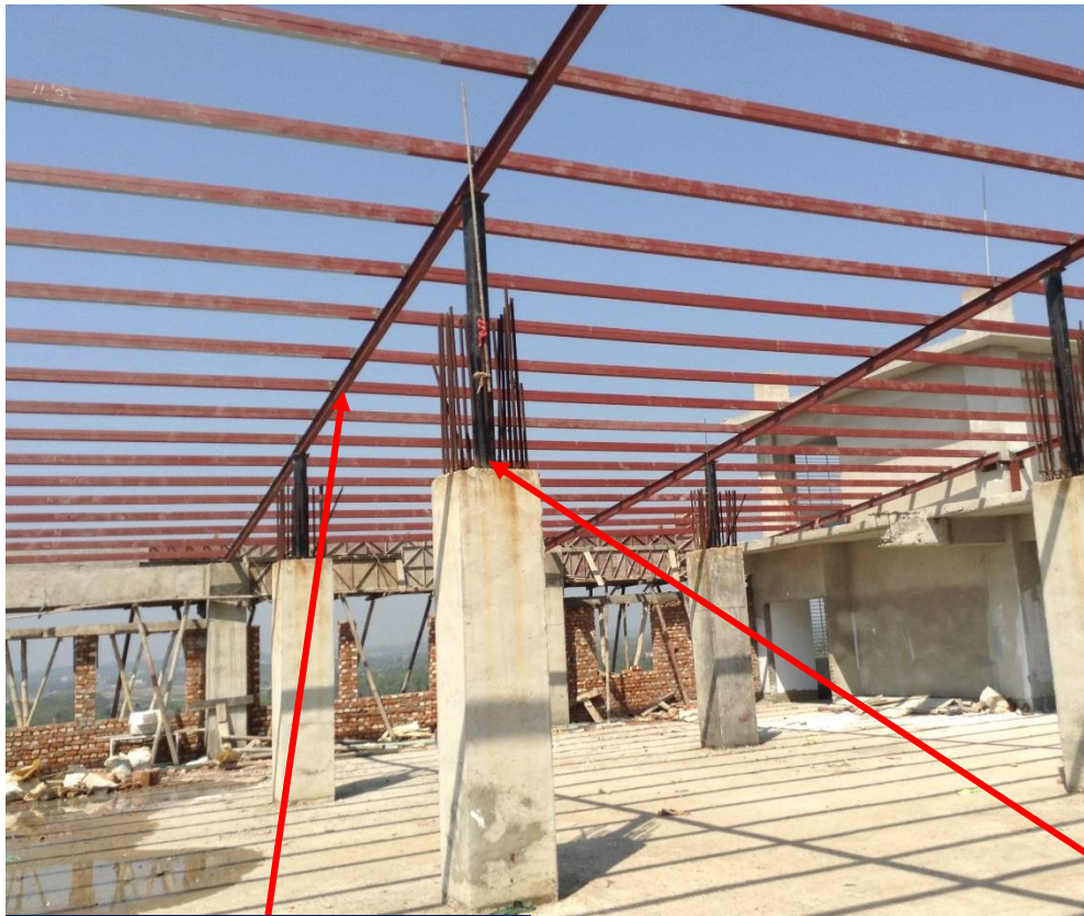
Roof beams appear slender
