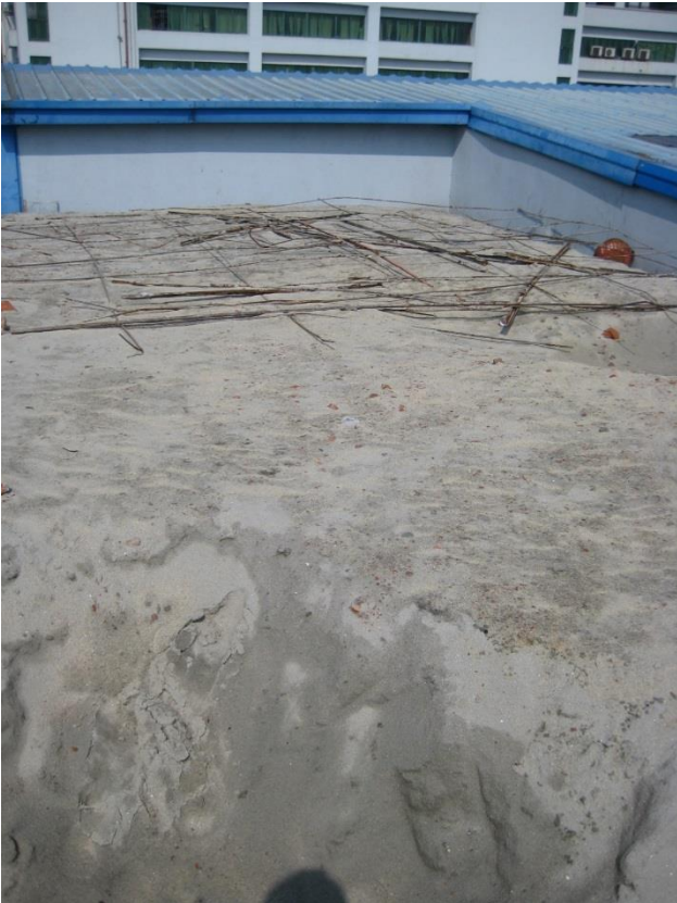
Sand on roof over east stair
