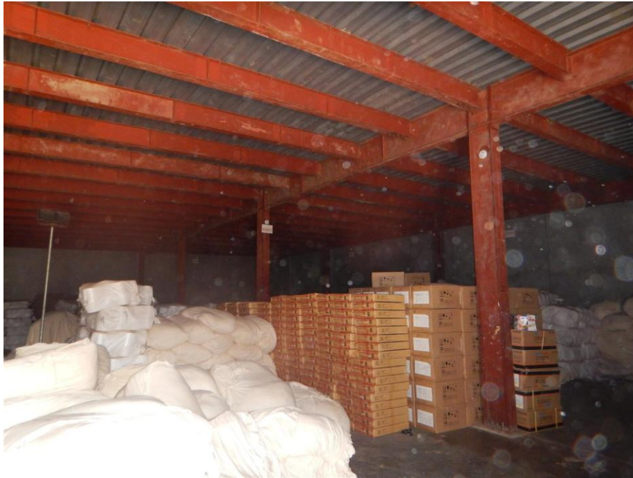
No visible fire protection to steelwork supporting first floor in Building 2.
