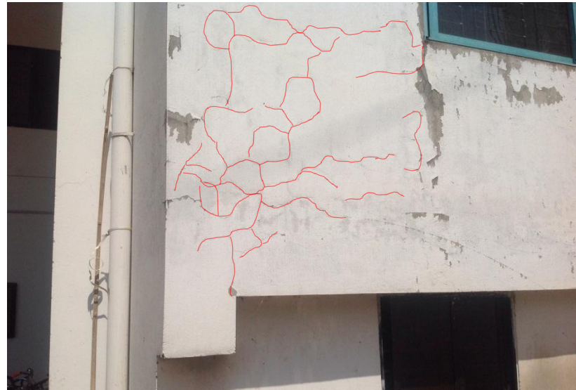
Cracking was noted in brickwork on exterior of stairwell
